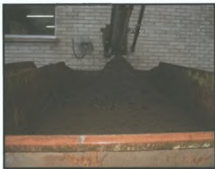
Figure 5.8 Sludge generated by belt press at Cavan wastewater treatment plant
