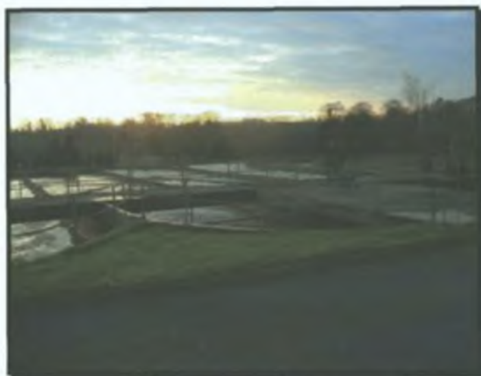
Figure 5.10 Extended aeration at Kilkenny wastewater treatment plant
