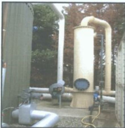
Plate: 5.7 Ammonia Scrubber
