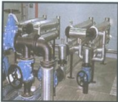
Plate:5.1 Heat exchanger unit
