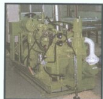
Plate:5.3 CHP unit
