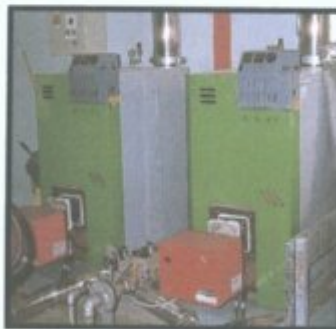
Plate:5.2 Gas boilers
