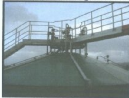
Plate: 5.4 External view of gas distribution pipes
