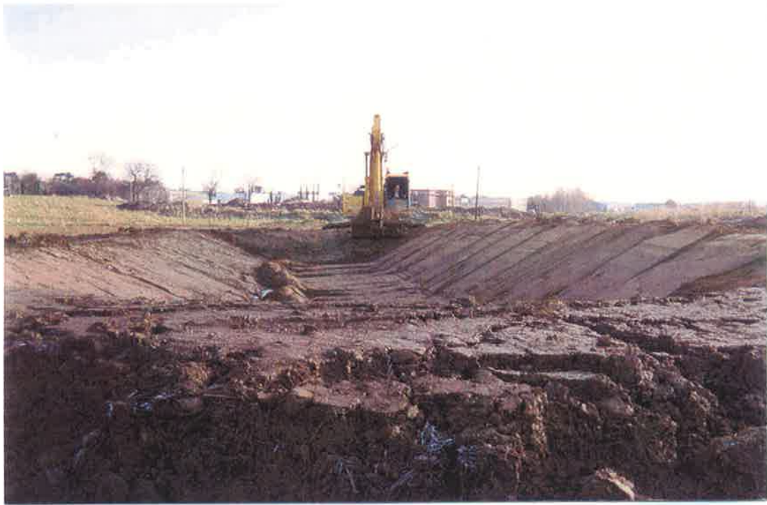
Fig. 3.3 Excavation of the TMF Wetland and placement of protective sand layer over the walls and base of the cell.
