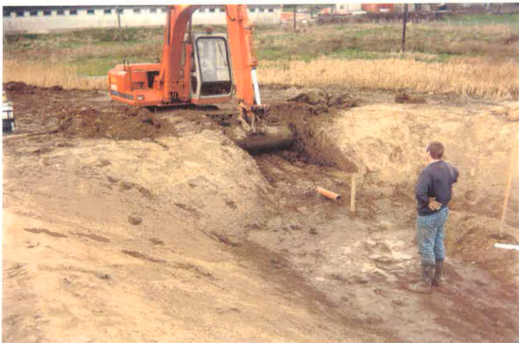
Fig. 3.4 Placement of outflow pipe and outlet controls in wetland cell to facilitate gravity flow.
