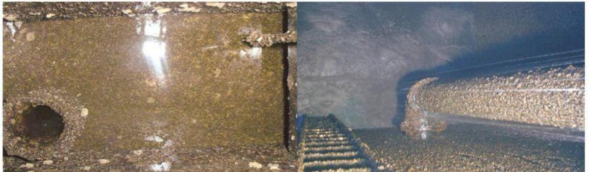
Figure 3.1 Zebra mussel infestation in raw water chambers at Sligo drinking water plant (photo by Eamon Fox).
