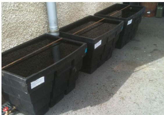
Figure 3.2 Bioboxes outside of Sligo drinking water treatment plant (photo by Sara Meehan).
