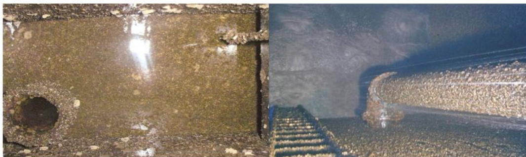
Figure 1. Zebra mussel infestation in raw water chambers at Sligo drinking water plant (photograph by Eamon Fox).
