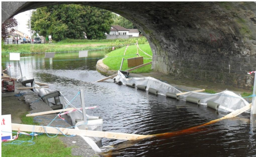
Figure 4.2 Impermeable curtains used to hold treated water within treatment area along canal walls (photo by Sara Meehan).
