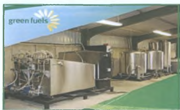
Figure 3.14 Ion exchange resin columns
