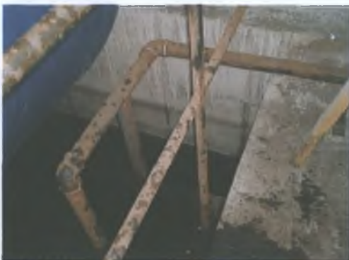
PLATE 4: TYPICAL BUND OBSERVED DURING AUDIT.
