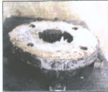
Gasket material adhering to a pipe flange
