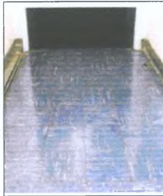
Asbestos-containing vinyl floor tiles
