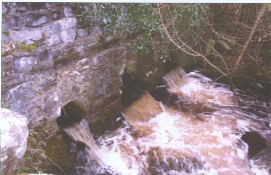
Plate 2.4 Round and box stone culverts on Yellow River, Co. Mayo (S. Neylon)
