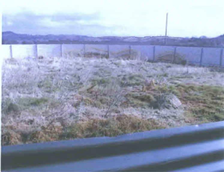
Plate 2.4 Interior of Drumaboden Puraflo system.
