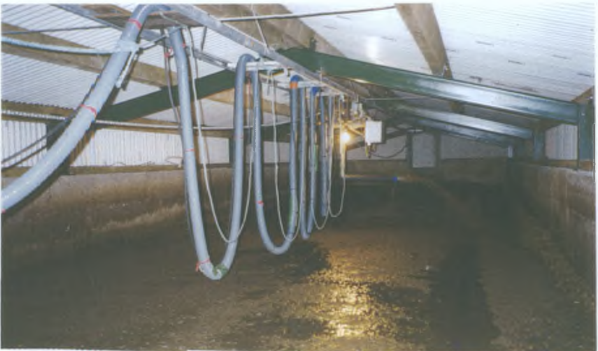
Plate 2.9: Internal View Of Liquid Vermicomposting Unit At Toomevara STP, Co. Tipperary.
