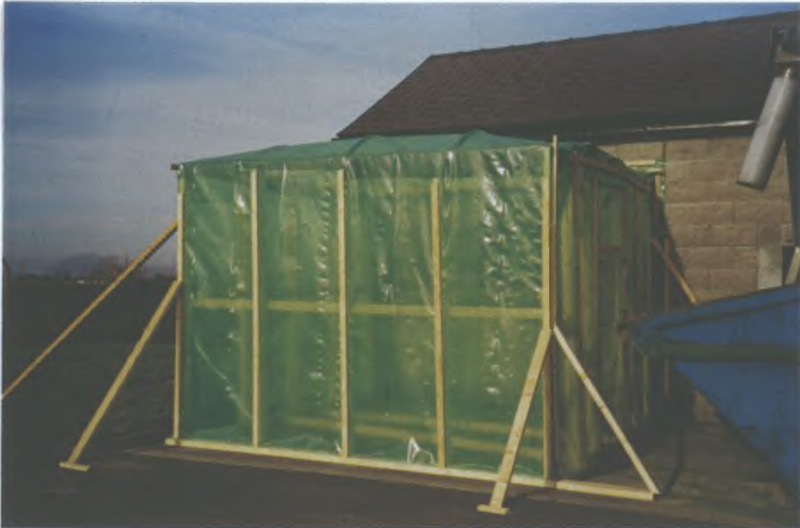
Plate 3.1: External View Of Vermicomposting Pilot Building At Bangor Erris Sewage Treatment Plant
