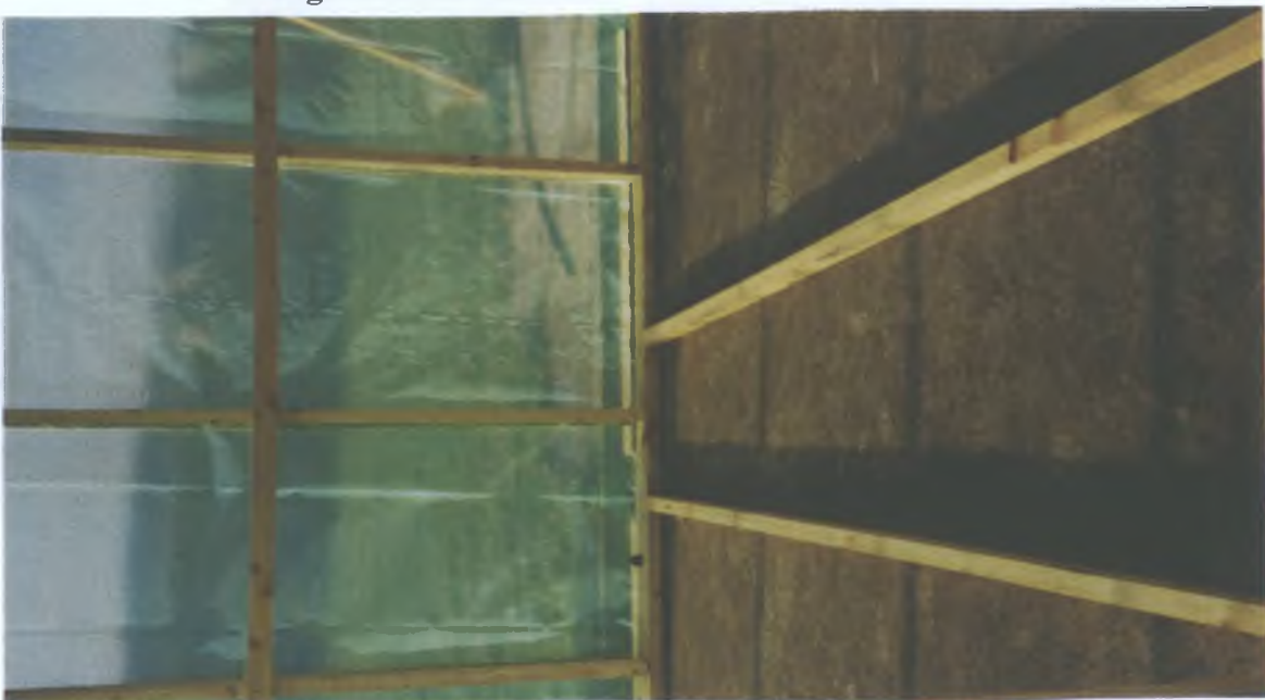
Plate 3.2: Internal View Of Vermicomposting Pilot Building At Bangor Erris Sewage Treatment Plant.
