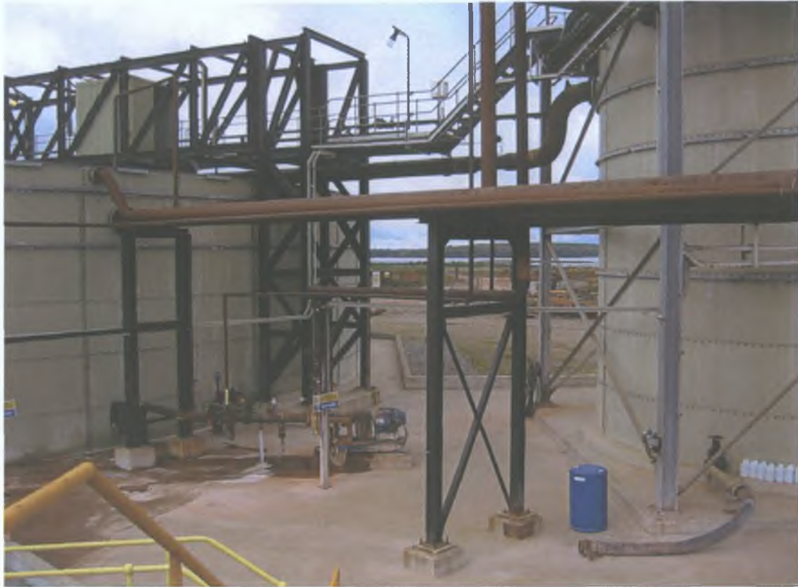
Plate 3.2 Clarifier on the right and buffer tank on the left with associated piping.
