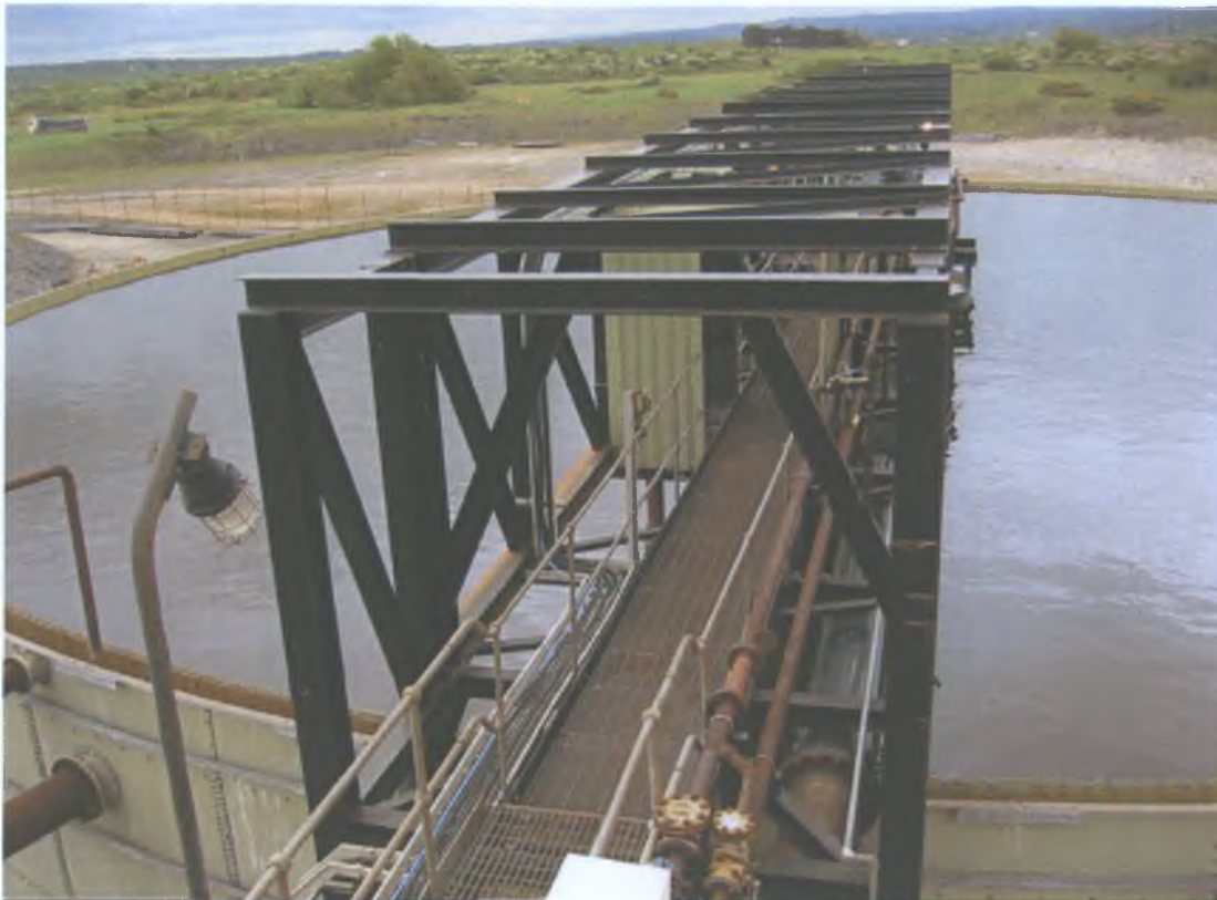
Plate 1.1 The 35 metre Clarifier at Aughinish Alumina.
