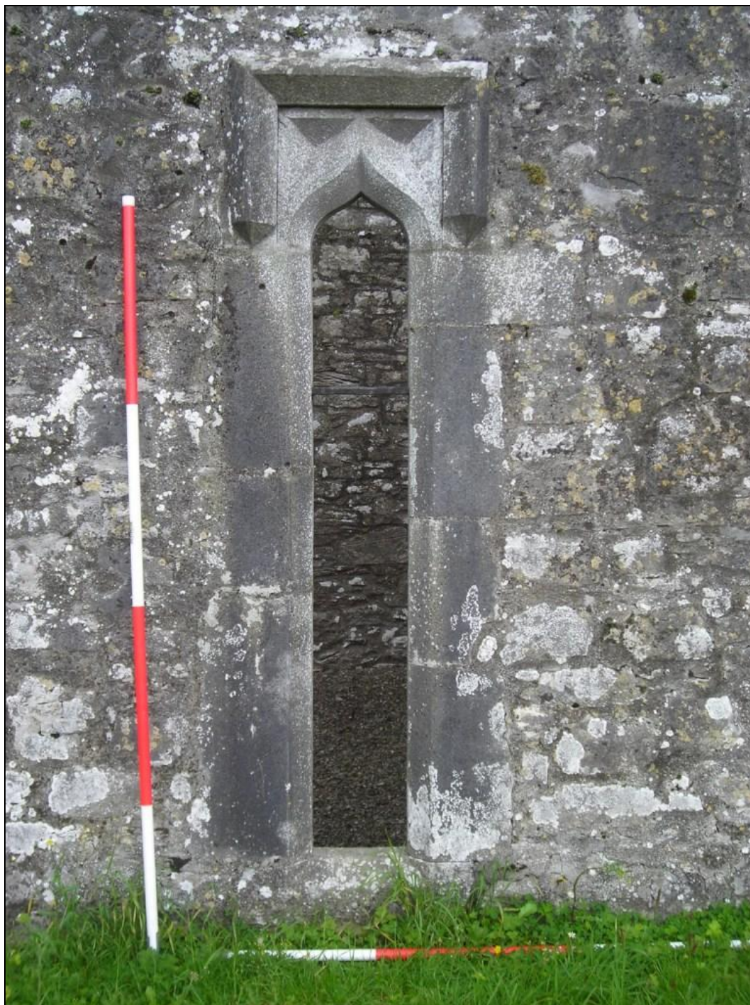
Figure 25: Single light window at rear of sedilia as seen from the exterior of the building
