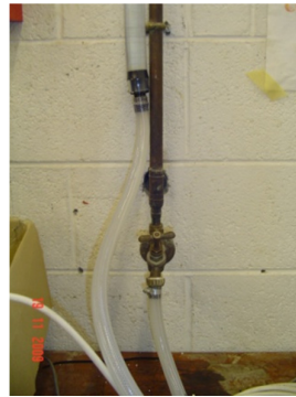
(a) Continuous water flow from rooftop reservoir
