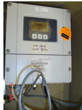
(c) Ultrasonic flow meter DAQ
