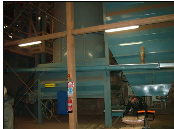
Figure 46: Chipping and grading line
