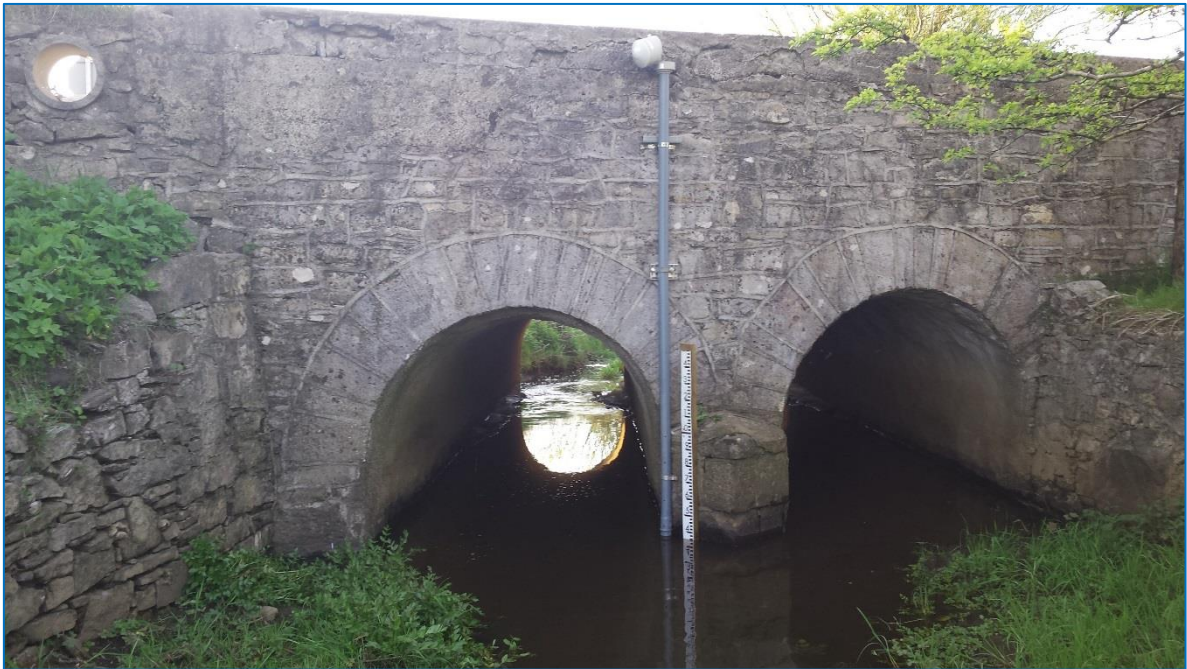
Figure 35: Hydrometric station installed at MP5 (Tullylinn) in early 2016
