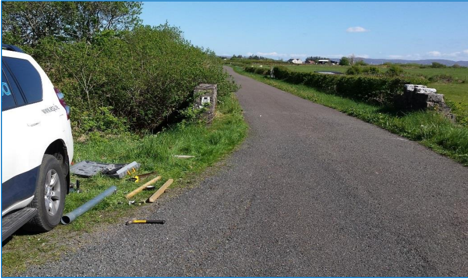
Figure 36: Construction & installation of new hydrometric station at MP6 (bridge in Stokane) – early 2016.
