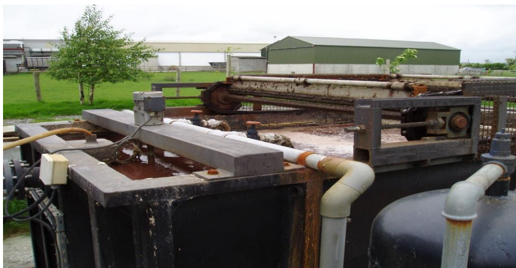
Figure 3.2: The DAF tank removing the white foam containing fat, oils and grease.
