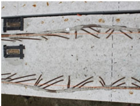
(b) lateral buckling of top chord (S29-14/07/06_2018)
