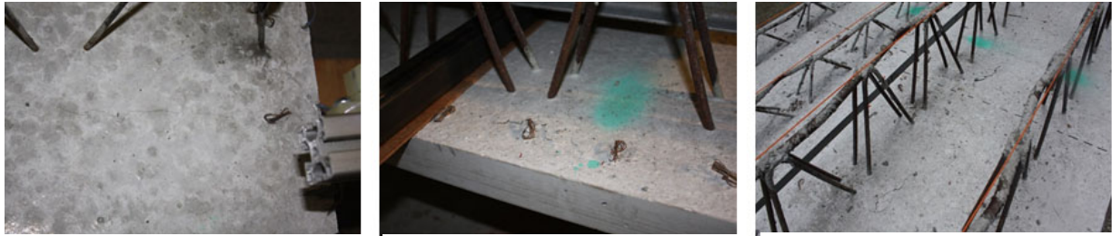
(a) Surface cracking between girders (W22.5-08/05/05)
