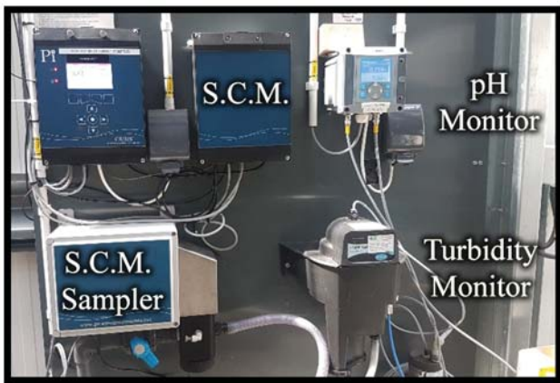
Figure 3. Wall mounted SCM
