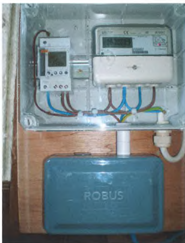
Figure 3.10: Elster A100C' single phase meter and Merlin Gerin 15720 electrical timer.
