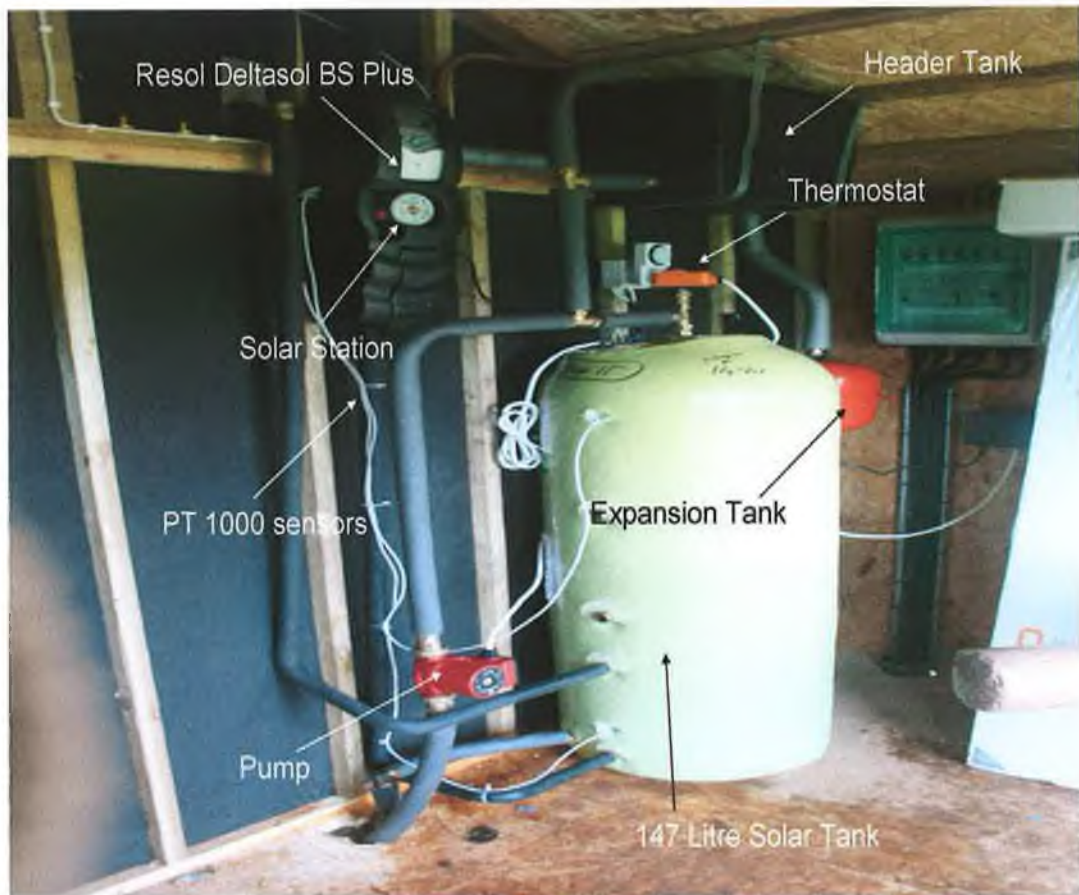
Figure 3.9: Solar Hot Water cylinder, solar station, expansion and header tanks.
