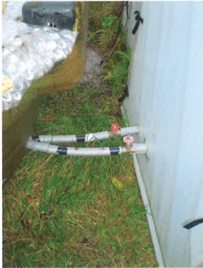
Figure 3.5: Brass gate valves connecting the inlet and outlet pipes of the HEU to the heat distribution system.
