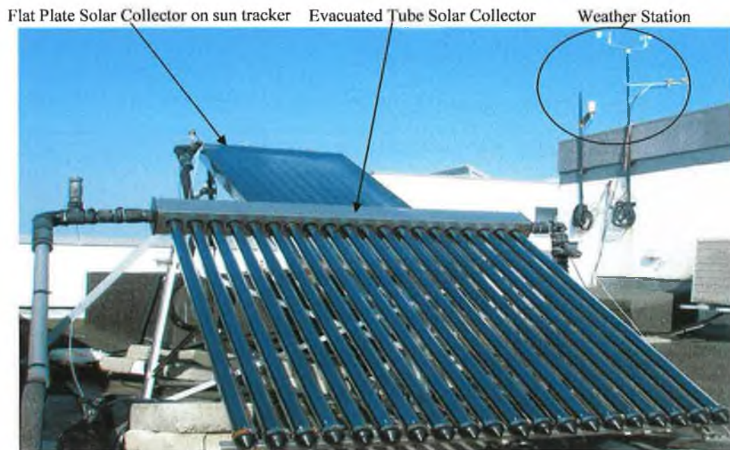
Figure 3.9 Photograph of Solar thermal collectors on the liBC building roof.
