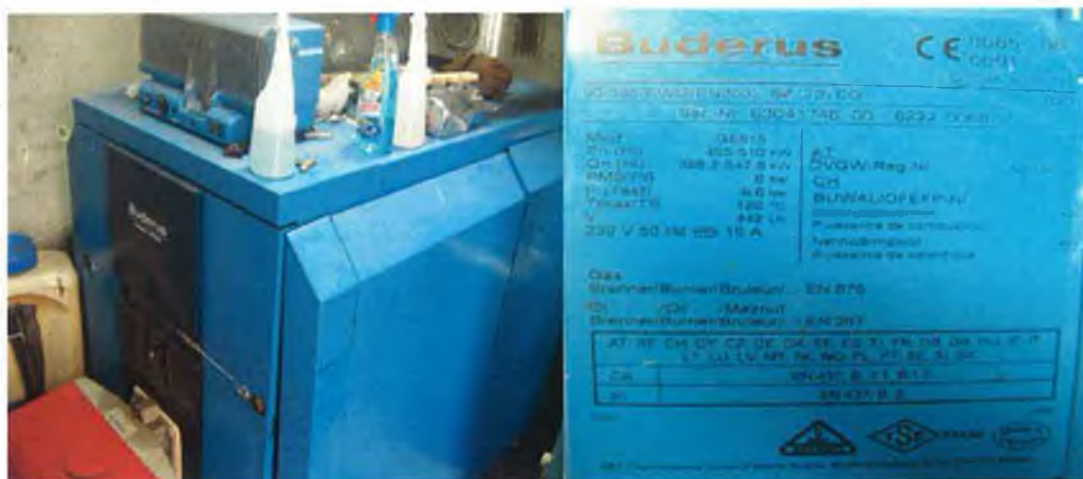
Figure 26: Boiler and Boiler Specification, Archbishop McHale College
