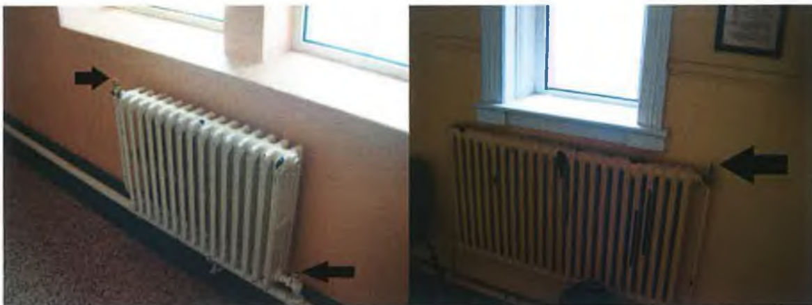
Figure 39: Radiator Valve Control Colaiste Cholmcille (left) and Archbishop McHale College (Right)
