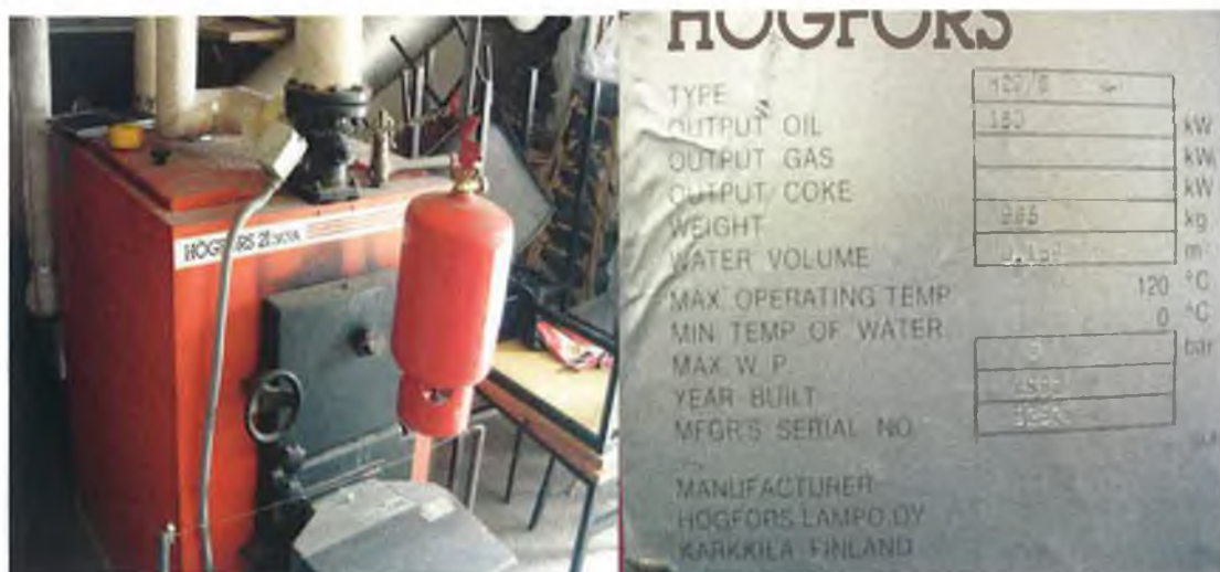
Figure 15: Boiler and Boiler specifications
