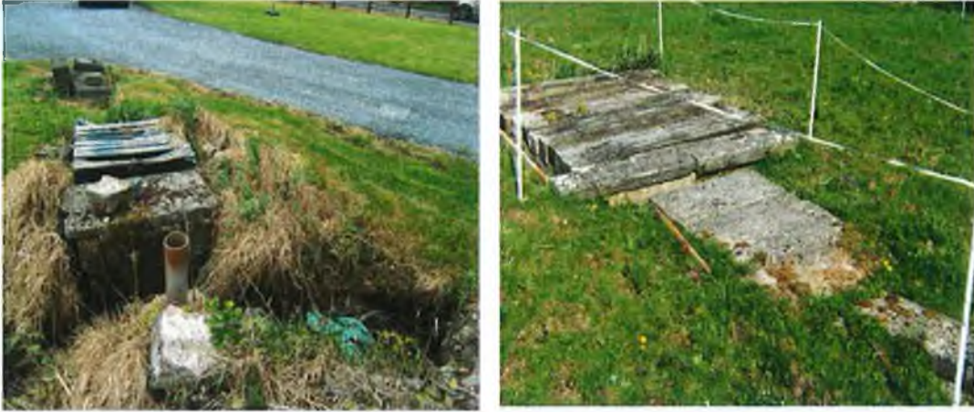
Plate 8.8: Inappropriate lids of septic tanks (O'Rourke, 2012).
