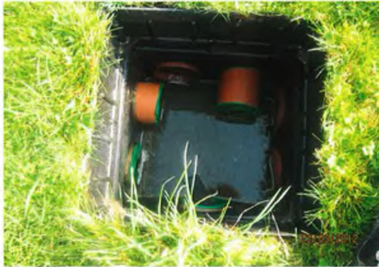
Plate 8.14: Properly installed distribution box (Cooney, 2012)
