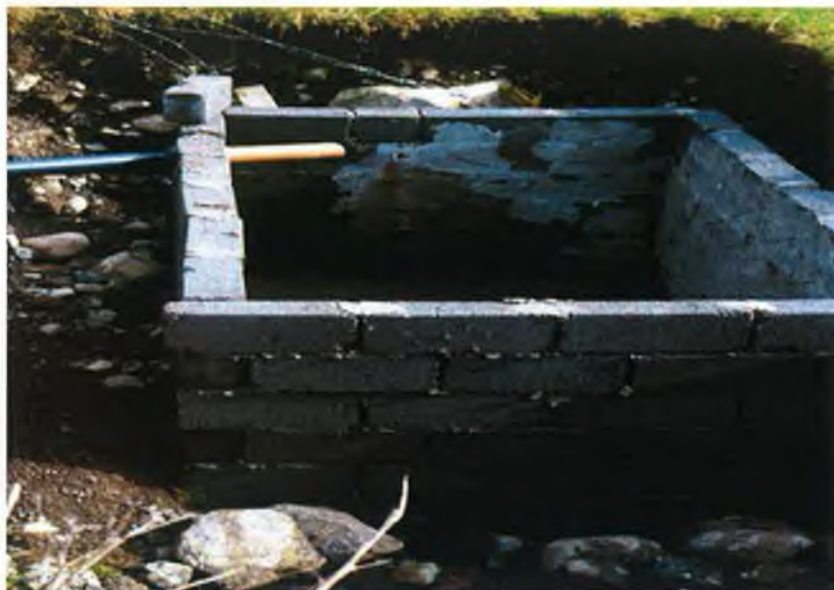
Plate 8.6: Poorly constructed Septic tank (Daly, 2005).
