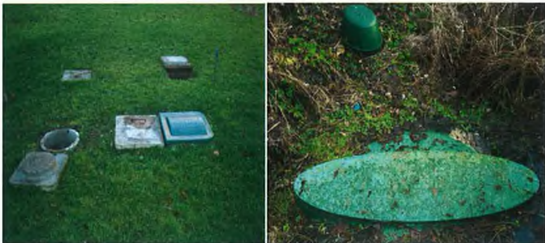
Plate 8.7: Oakstown BAF, Kingspan RBC Secondary Treatment Systems
