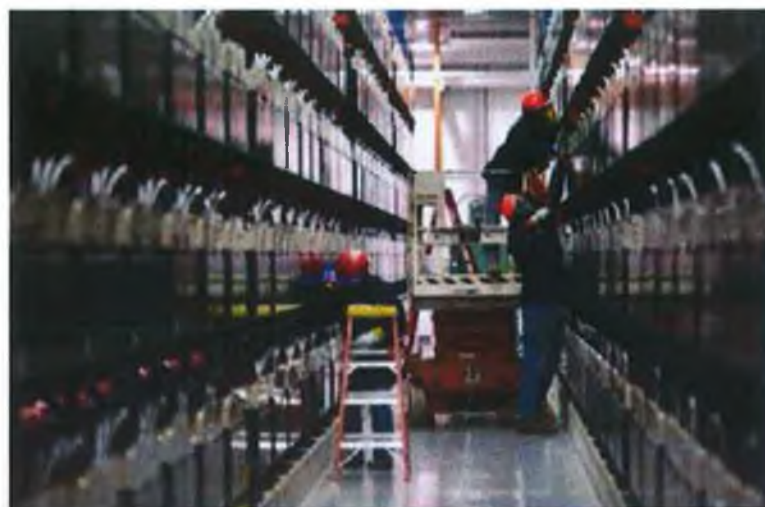
Figure 2.13 BESS at Golden Valley Alaska (Baker, 2008)
