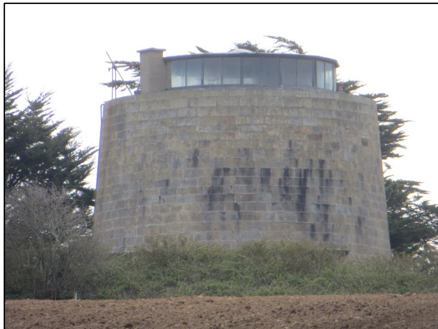
Figure 2.9. Duncannon Martello Tower North (Reg. No. 15704413) located on raised ground to the north-east of Duncannon Fort, County Wexford. The tower has been converted into residence.
