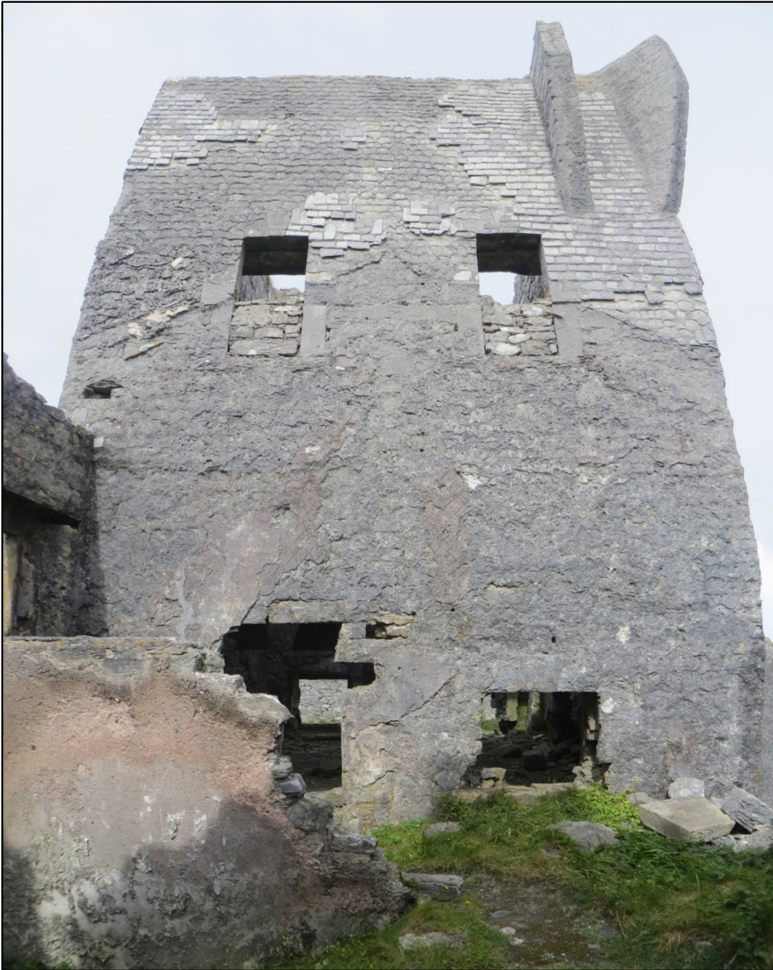
Figure 3.8. This image of the south-east wall of the signal tower on Inishmore, County Galway, is a compilation of several images joined together in Panorama Maker 6 . It displays extreme curvature of the walls beyond the level that could be adjusted for using the Barrel Distortion Correction tool in PaintShop Pro X8 . The presence of abutting buildings meant that the photographs could not be taken at a more appropriate distance from the wall.
