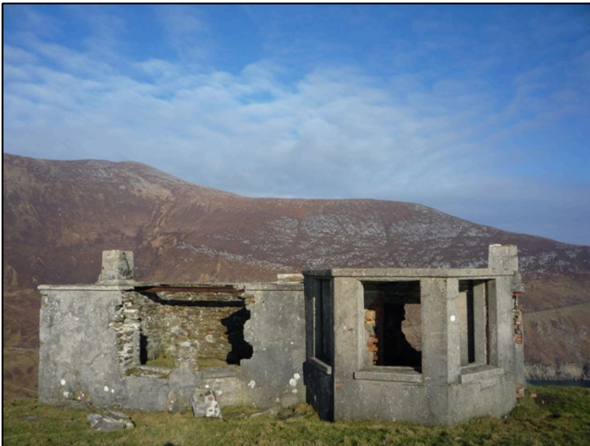
Figure 4.52. The early 20th century watch house at Moyteogue, Achill Island, County Mayo, looking north-east.
