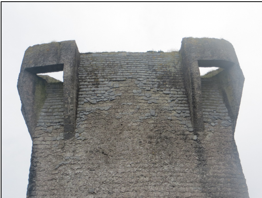
Figure A.8. The parapet level of the north-east wall showing the bartizans and patches of weather-proof slates.
