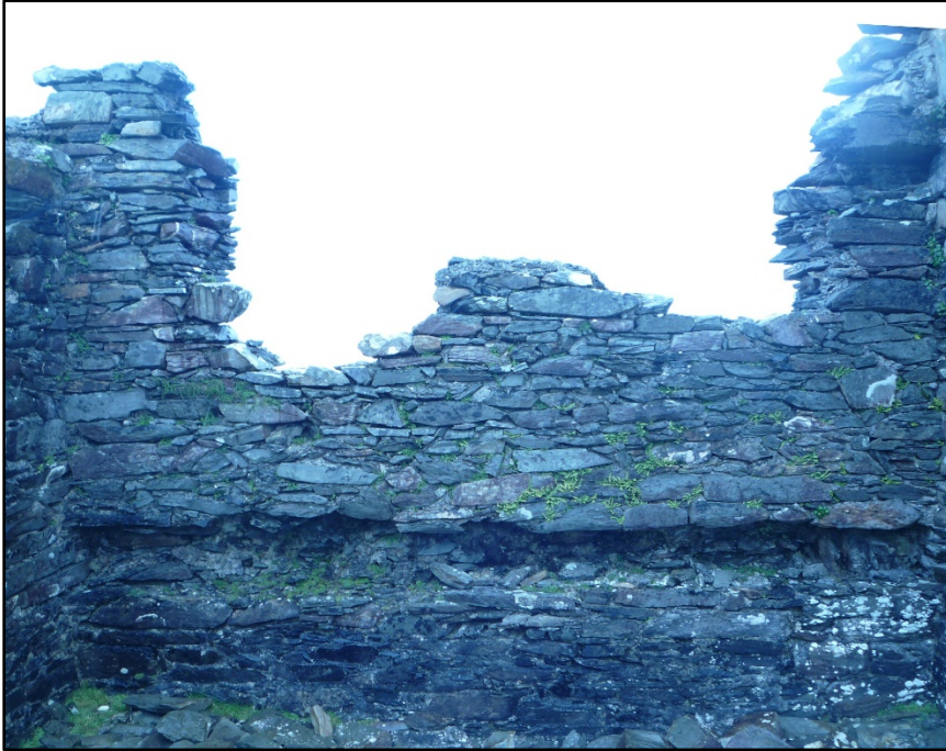
Figure B.10. The internal face of the north wall of the signal tower at Inishturk Signal Station.
