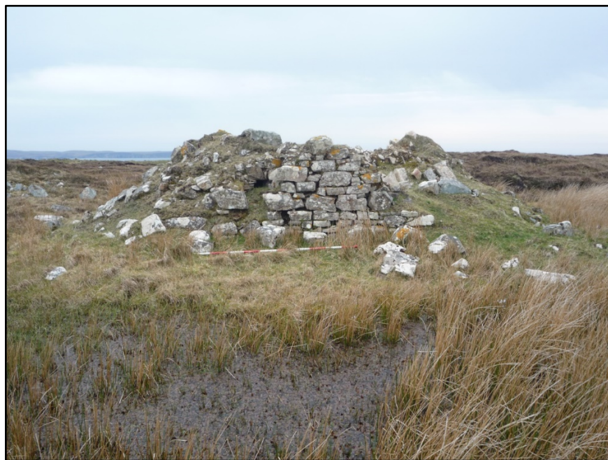
Figure B.78. The east side of the signal tower at Benwee Head Signal Station.
