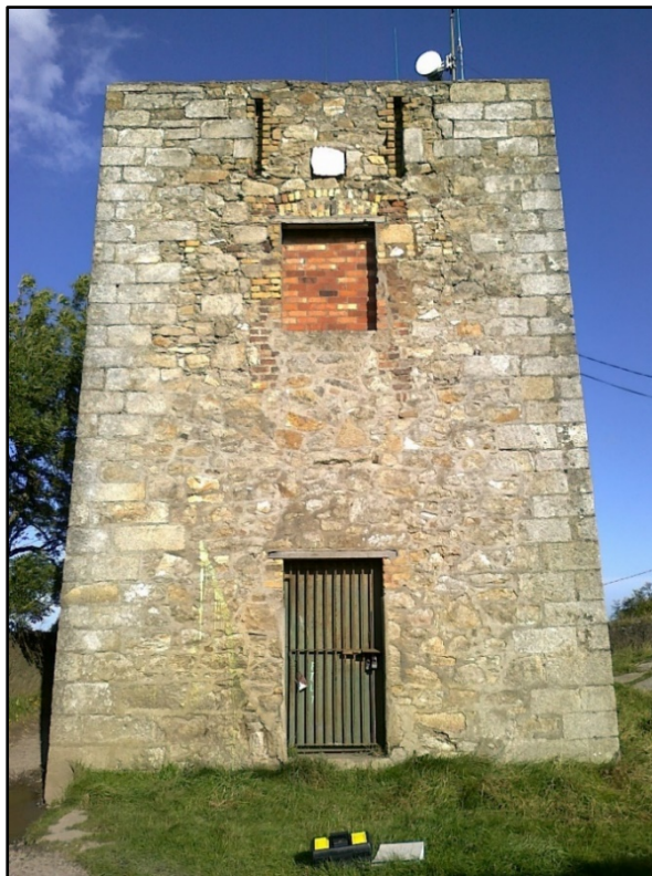
Figure E.4. The south-west wall of the signal tower at Dalkey Signal Station, County Dublin, looking north-east. (Photograph courtesy of Gary Dempsey).
