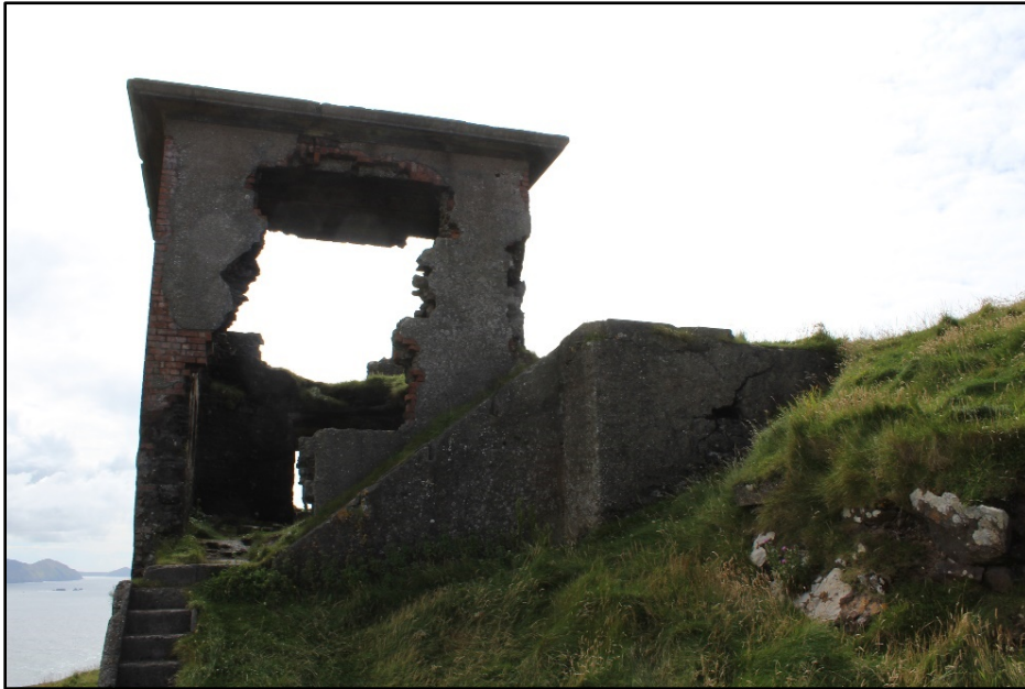
Figure F.30. View of the north-east side wall of the two storey building at Sybil Head Signal Station, County Kerry, looking south-west, with steps in the foreground. (Photograph courtesy of Dr James Bonsall).
