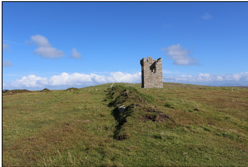
Figure B.54. The west wall of the signal tower at Glash Signal Station.
