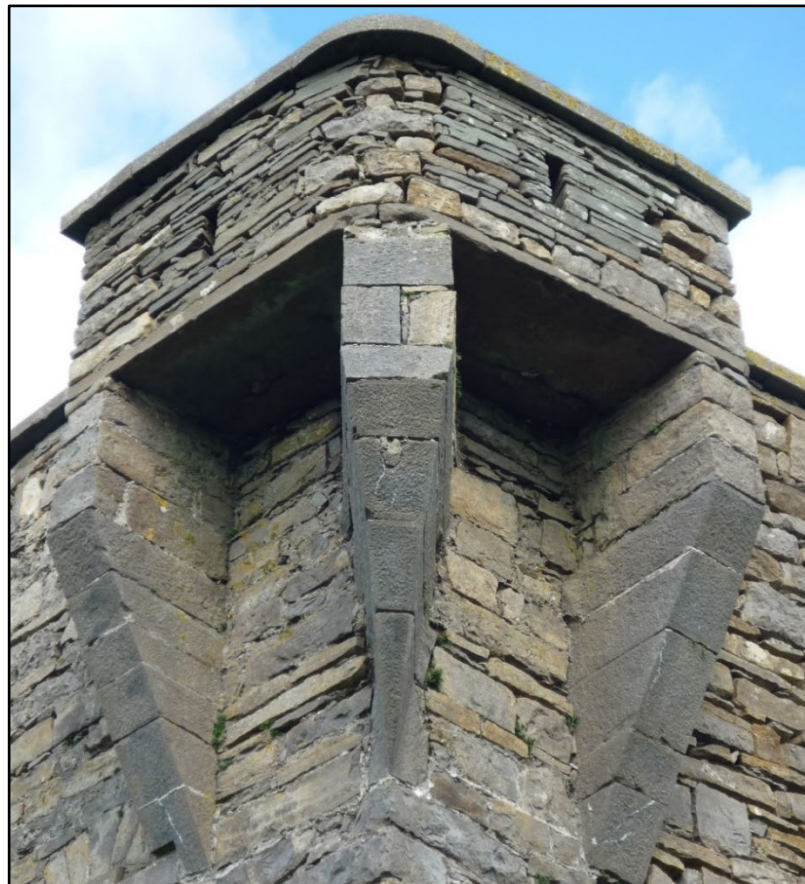
Figure C.50. Detail of the bartizan at the signal tower at Carrowmably Signal Station, showing the two outward facing gun-loops.
