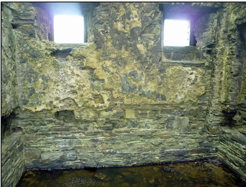
Figure D.30. The lower portion of the internal face of the north-west wall of the signal tower at Carrigan Head Signal Station. The row of three holes in the side stone of the south window which would have held horizontal bars protecting the window are visible towards the top right of the image.
