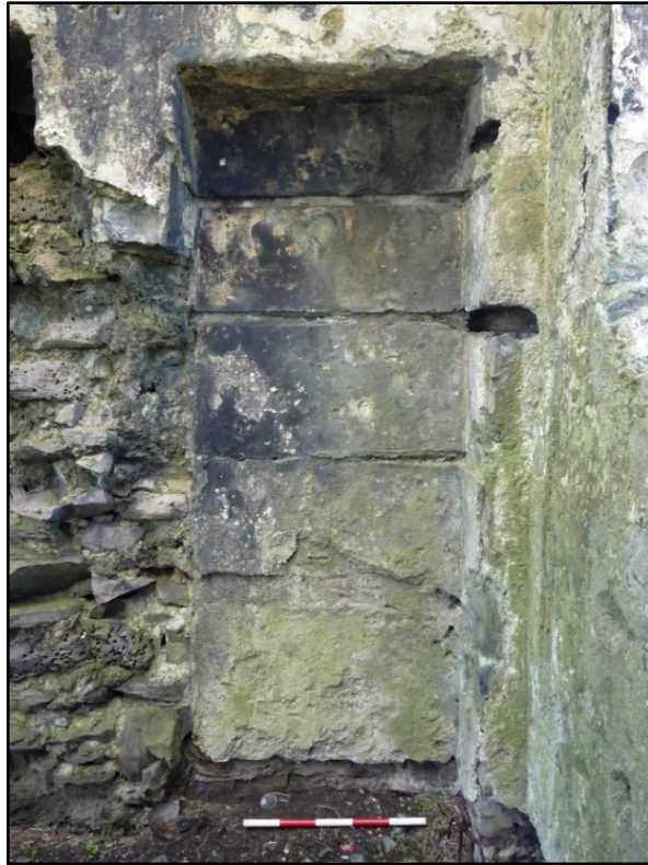
Figure C.22. The east alcove in the ground floor level of the internal south wall face showing the impression of four shelves in the render.
