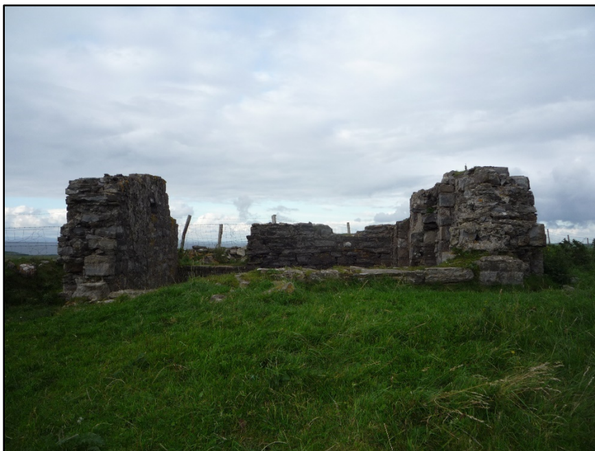
Figure C.63. External face of the south-west wall of the collapsed signal tower at Knocklane Hill Signal Station.
