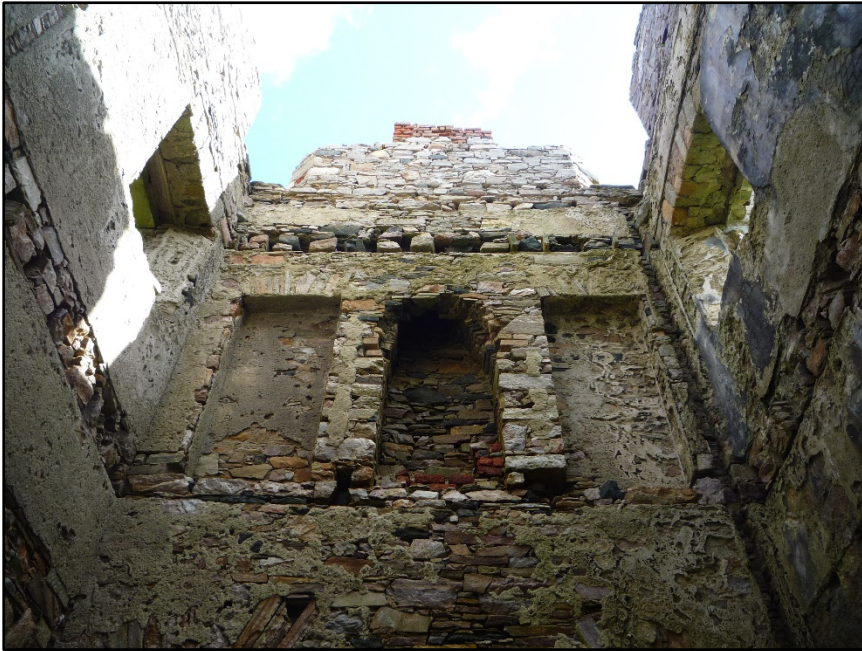
Figure D.59. The upper portion of the internal face of the south-east wall of the signal tower at Crohy Head Signal Station.
