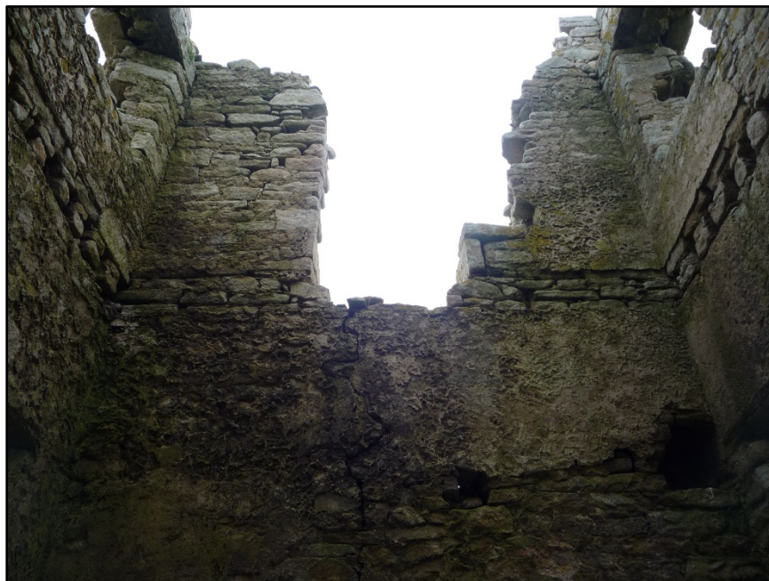
Figure B.56. The upper part of the internal wall face of the west wall of the signal tower at Glash Signal Station, showing the badly damaged first floor door.
