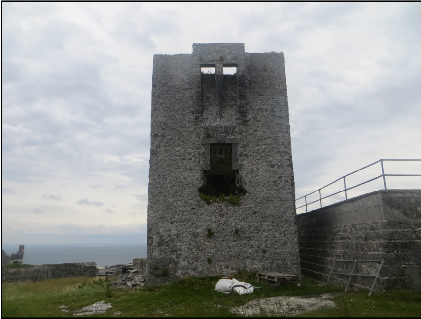
Figure A.7. View of the south-west wall of the signal tower, showing the first floor door and the machicolation which protected it. Note the absence of the stone surround on the lower half of the door.
