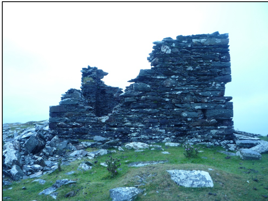
Figure B.9. The external face of the east wall of the signal tower at Inishturk Signal Station.
