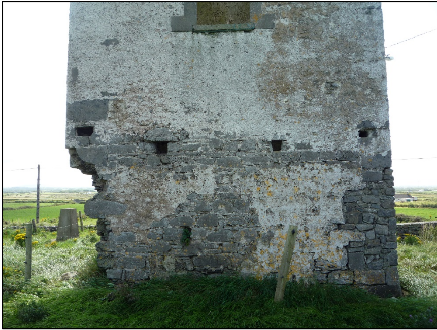
Figure C.20. The lower part of the external face of the north wall of the signal tower at Rathlee Signal Station. The bottom of the door can be seen, above the uneven row of four holes penetrating into or passing through the body of the wall. The damaged north-east corner can be seen at the left.
