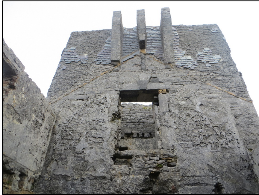
Figure A.28. The upper part of the south-west wall of the signal tower, showing the first floor door, the corbels and piers of the machicolation reaching the reduced top of the parapet wall, patches of weather-proof slate and the impression of the roof line of the two storey south-west addition.
