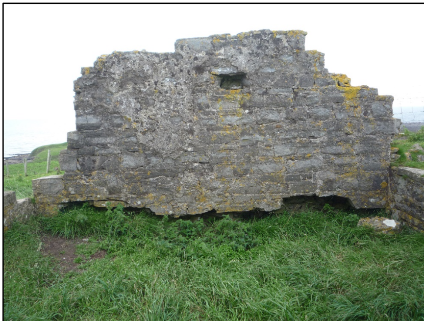
Figure C.65. Internal face of the north-west wall of the collapsed signal tower at Knocklane Hill Signal Station. The slot for the ground floor level can be seen at the bottom of the exposed section of wall.
