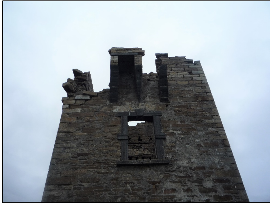
Figure D.41. The upper portion of the external face of the north-west wall of the signal tower at Glen Head Signal Station, showing the first floor doorway with its intact stone surround and the partially collapsed machicolation.
