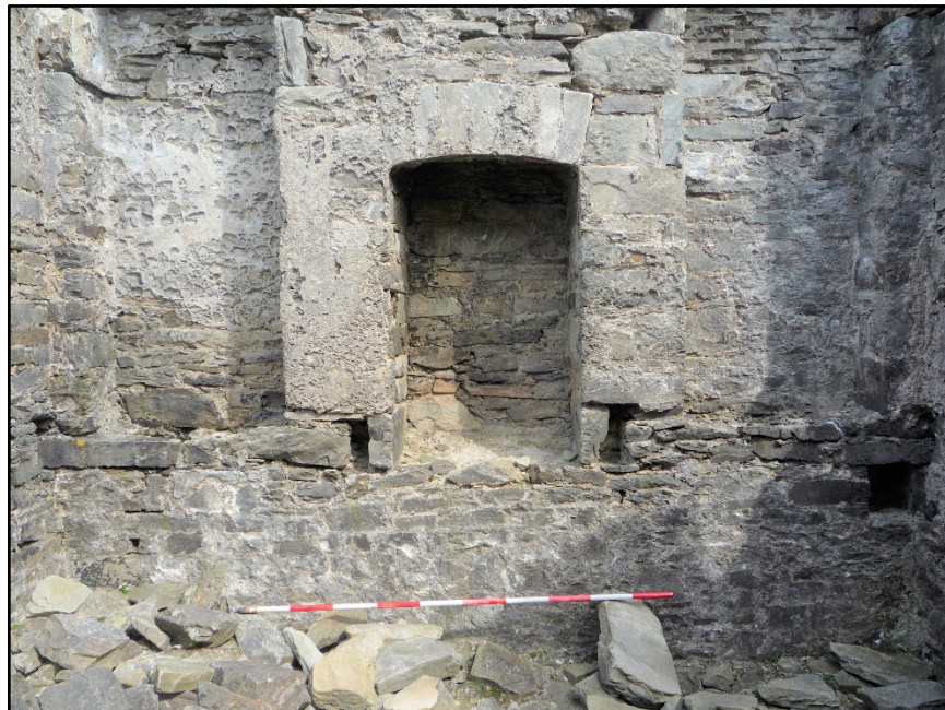
Figure B.39. View of the internal face of the west wall of the signal tower at Saddle Hill Signal Station, showing the ground floor central fireplace and the flanking alcoves. The horizontal chute can be seen at the right of the image, at the top of the semi-basement level.
