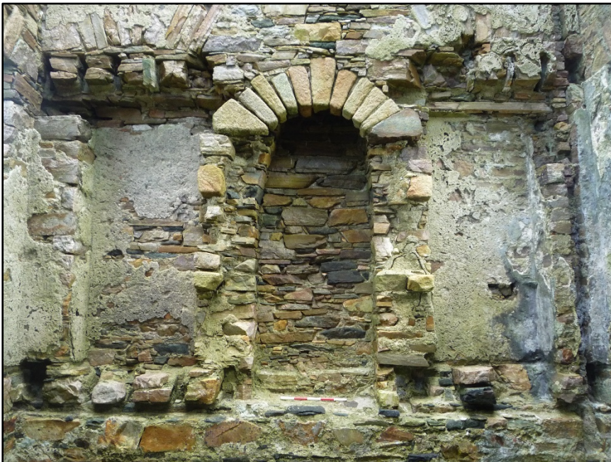
Figure D.60. The lower portion of the internal face of the south-east wall of the signal tower at Crohy Head Signal Station, showing the slot with joists holes for the ground floor, the ground floor central fireplace and the flanking alcoves, and the joist holes of the split mezzanine level.
