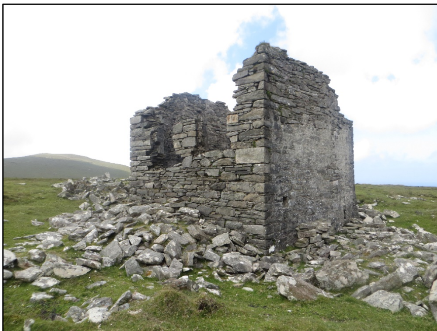
Figure B.37. View of south-east corner of the signal tower at Saddle Hill Signal Station.
