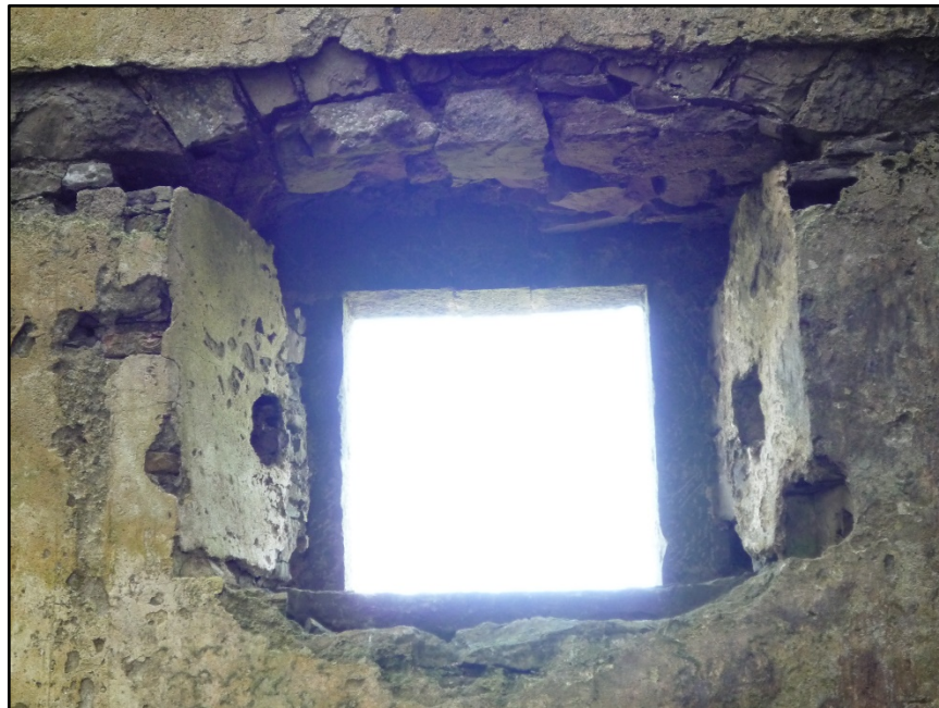
Figure C.46. Interior detail of the north ground floor window on the west wall, showing the large holes on the splayed sides of the window which may have held a wide horizontal timber.
