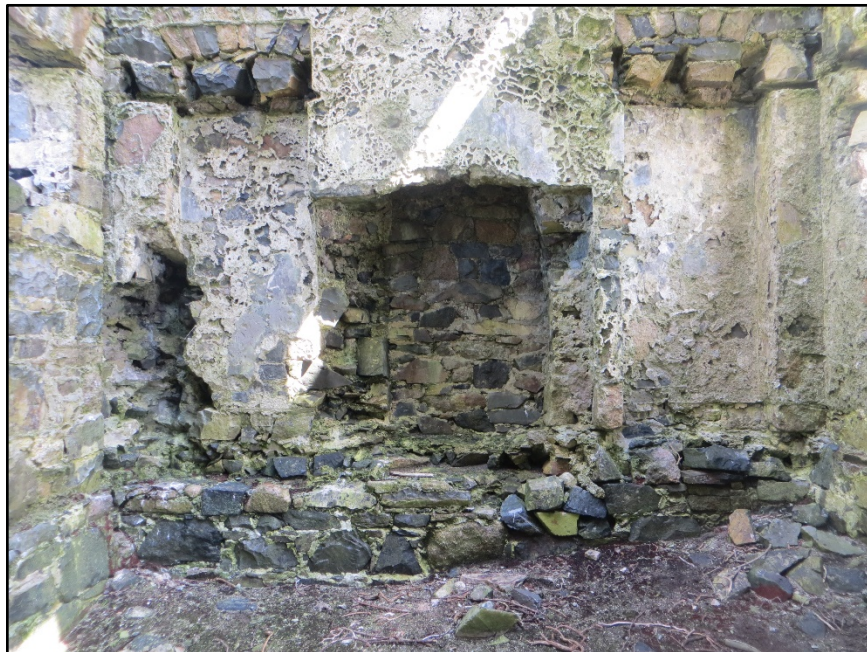
Figure A.58. The lower portion of the internal face of the north-east wall, showing the central fireplace flanked by alcoves and the joist holes of the split mezzanine level.
