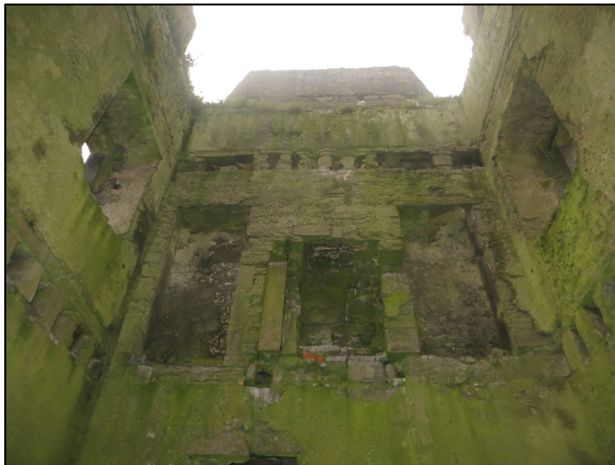
Figure A.10. The first floor and parapet level of the internal face of the north-east wall, showing the first floor alcoves and fireplace, the joist holes of the attic level, the instep at the parapet level for the roof, and the entrances to the two bartizans.
