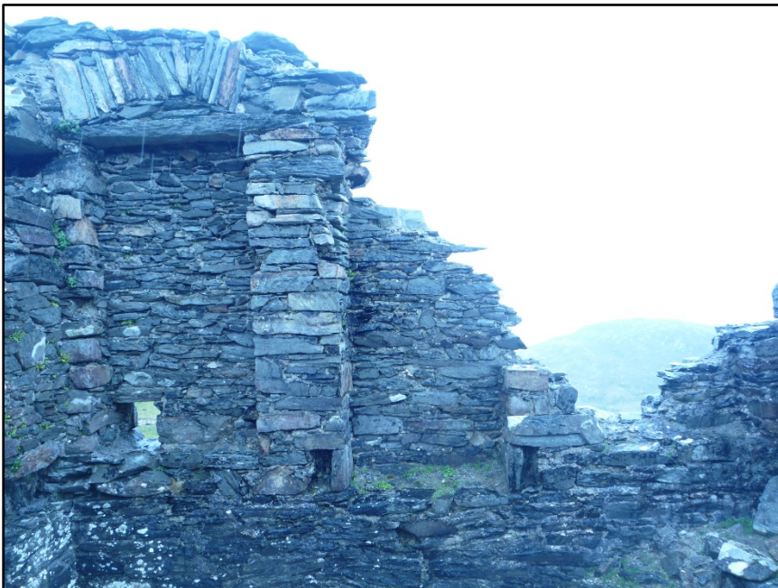
Figure B.11. The internal face of the east wall of the signal tower at Inishturk Signal Station, showing the intact north alcove with the square chute at its north edge, the damaged central fireplace and the fragments of the south alcove.
