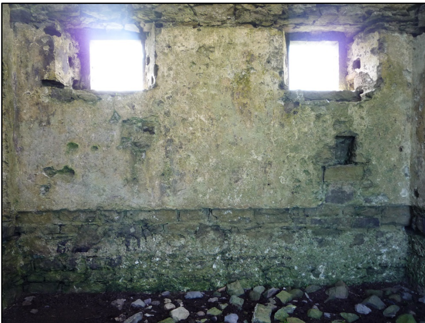
Figure C.44. The lower portion of the internal wall face of the south wall of the signal tower at Carrowmably Signal Station. The un-rendered semi basement level, the rectangular hole under the north window and the ground floor windows with square bar holes are visible.
