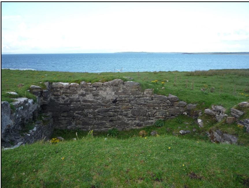
Figure C.76. The internal north-east wall face of the collapsed signal tower at Streedagh Signal Station.
