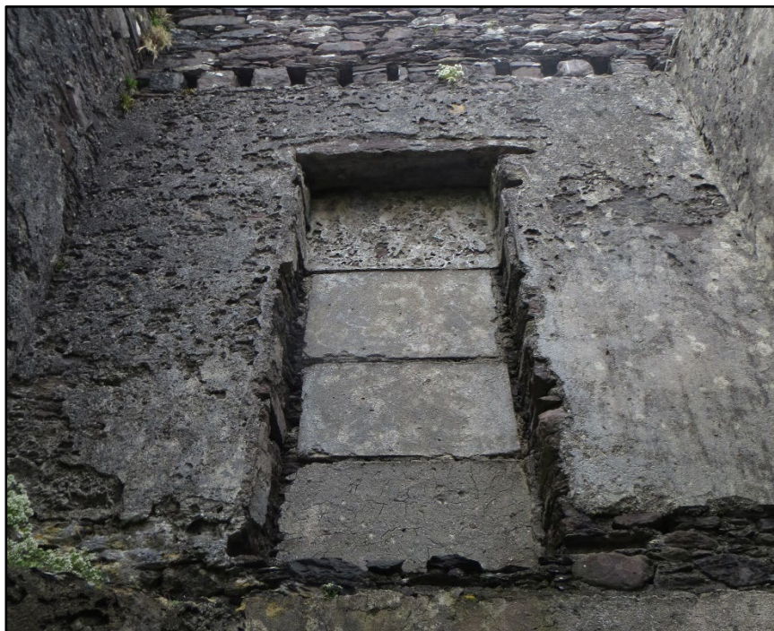
Figure G.7. Alcove with shelf impressions on the first floor of the building.
