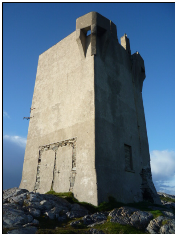
Figure D.120. The south corner of the modified signal tower at Malin Head Signal Station.
