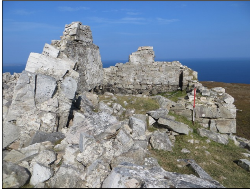
Figure A.91. View of the collapsed west wall with the internal face of the north wall of the collapsed signal tower at Cleggan Hill Signal Station in the background.
