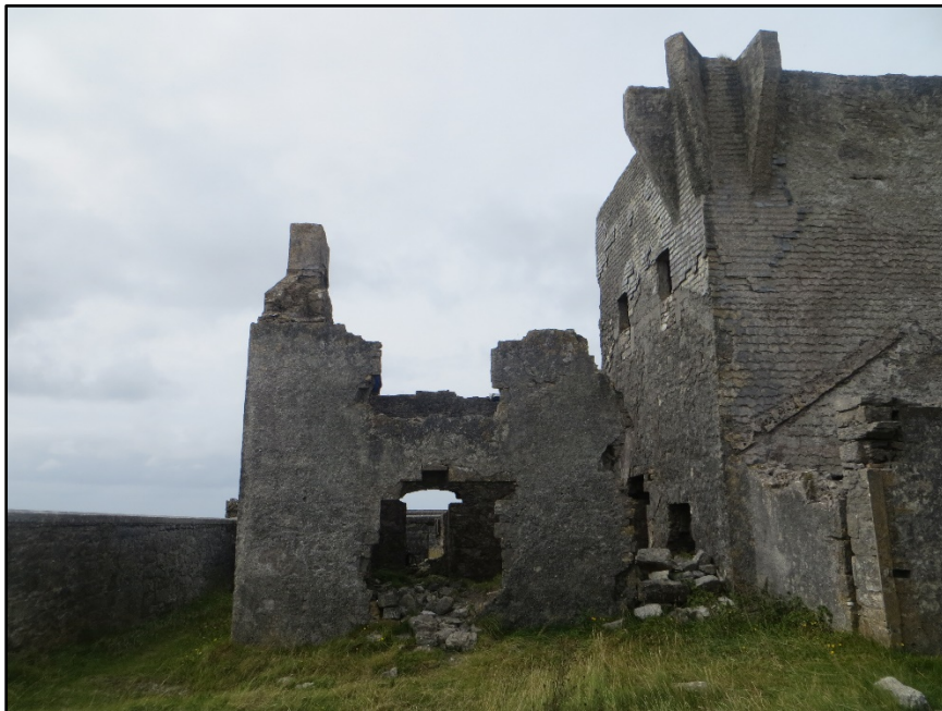
Figure A.35. The north-east wall of the one and a half storey addition to the south-east of the signal tower, with the chimney on the end wall visible at the left of the picture.
