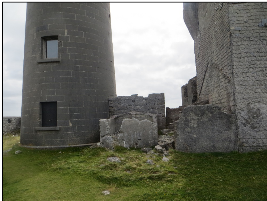
Figure A.37. The demolished and altered remains of the north-east addition, between the signal tower and the cylindrical lighthouse.
