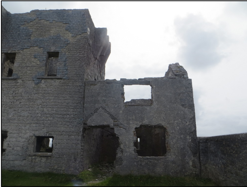
Figure A.34. The north-west wall of the two storey addition to the south-west of the signal tower, with the impression of the porch over the entrance visible on the wall adjacent to the signal tower.
