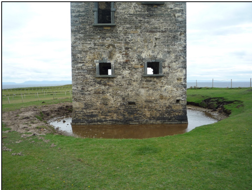
Figure D.26. The lower portion of the north-west external wall of the signal tower at Carrigan Head Signal Station, showing the water filled hollow around the signal tower.
