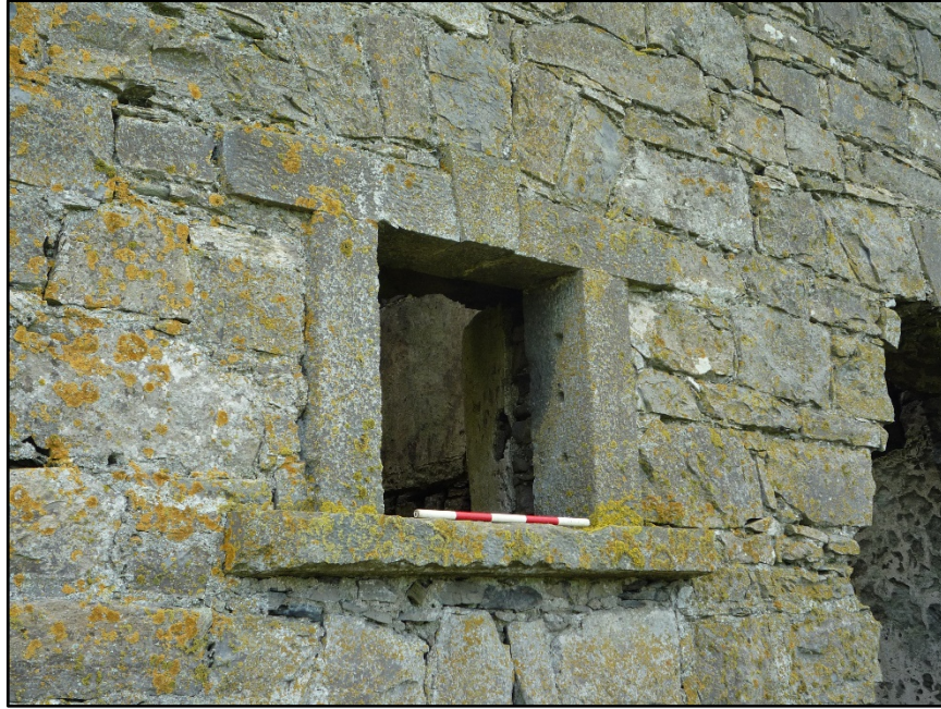
Figure C.45. Exterior detail of the south ground floor window on the east wall, showing the intact stone surround and the three small holes for window bars in the side stone.
