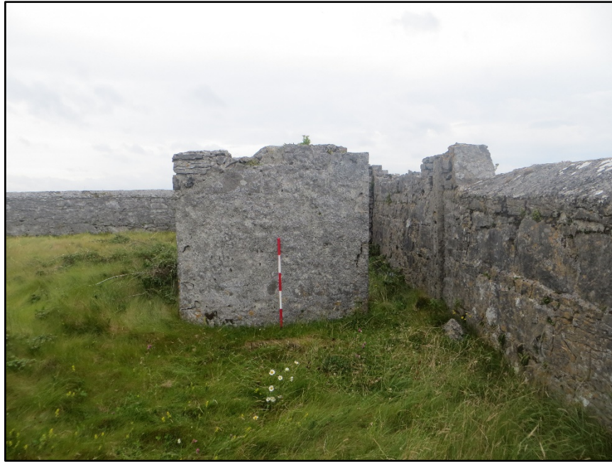
Figure A.13. The north-west side wall of the toilet block, with the door opening to the right. He enclosure wall was used as the rear wall of the building.
