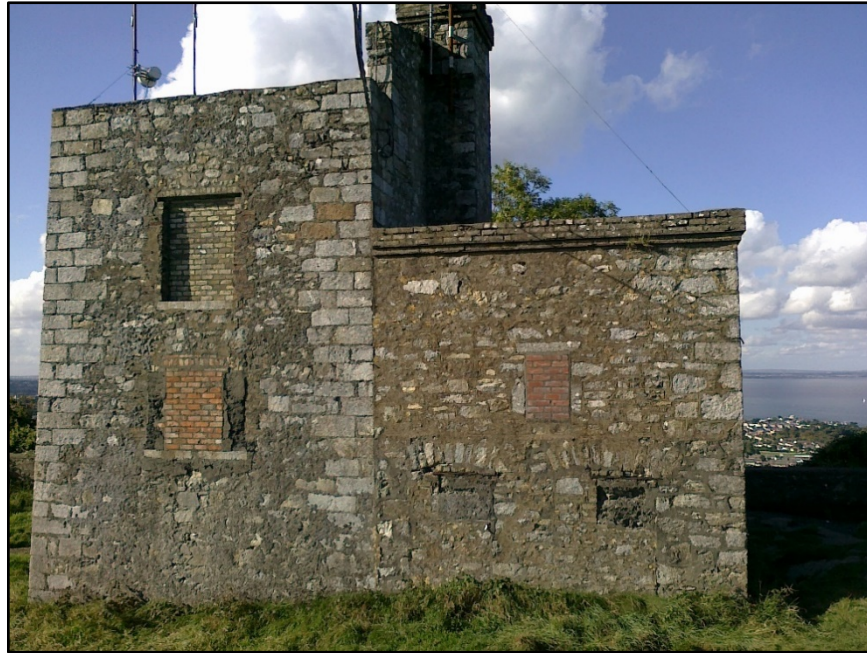
Figure E.5. The south-east wall of the signal tower at Dalkey Signal Station, County Dublin, showing the addition, looking north-west. (Photograph courtesy of Gary Dempsey).
