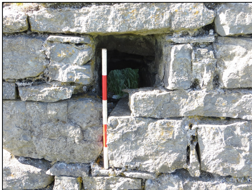
Figure C.10. Detail of the chute passing through the south-east wall of the signal tower at Lenadoon Point Signal Station.
