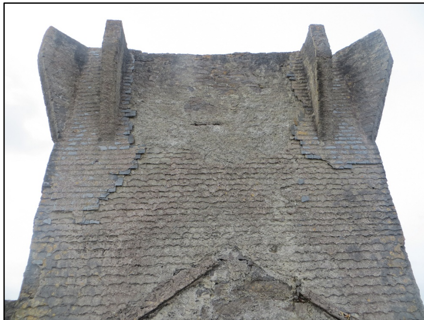
Figure A.29. The upper part of the north-east wall of the signal tower, showing the corbels and piers of the bartizans reaching the reduced top of the parapet wall, patches of weather-proof slate and the impression of the roof line of the single storey north-east addition.
