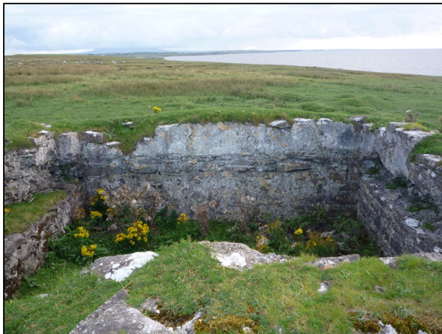
Figure C.78. The internal south-west wall face of the collapsed signal tower at Streedagh Signal Station.
