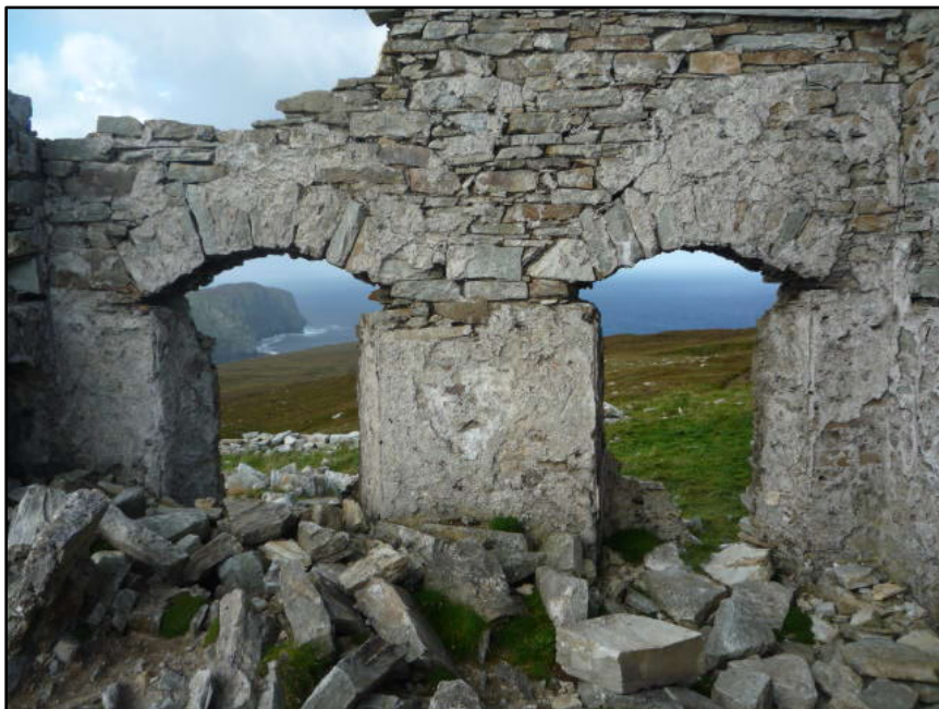
Figure D.92. The lower portion of the internal face of the west wall of the signal tower at Horn Head Signal Station, showing the ground floor windows with their unusual arched tops.
