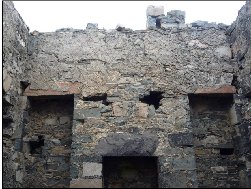
Figure B.21. The upper part of the internal face of the east wall, showing the top of the fireplace and the flanking alcoves.
