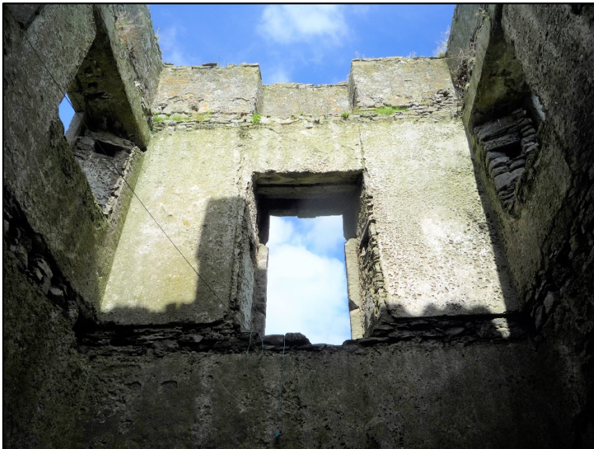
Figure C.25. Interior detail of the door on the north wall, showing the impression of the first floor and parapet level roof, above which is the entrance to the machicolation over the door.
