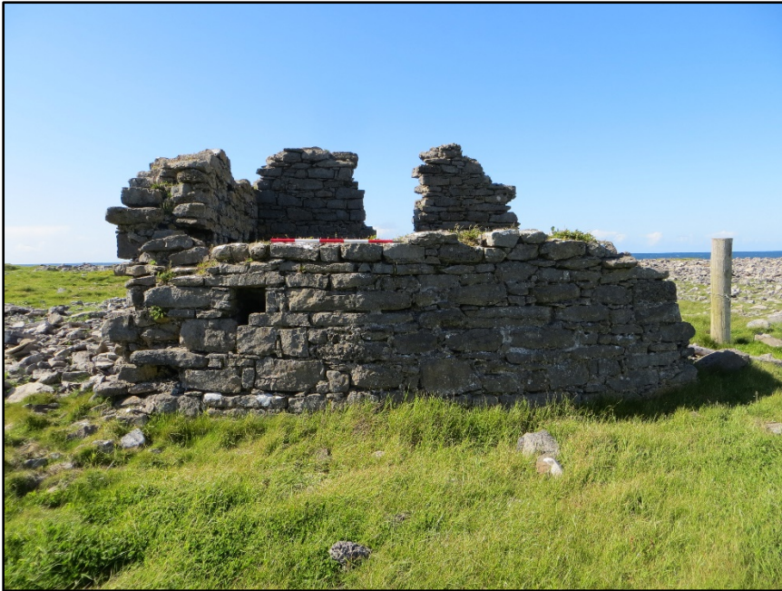
Figure C.7. View of the external face of the south-east wall of the collapsed or unfinished signal tower at Lenadoon Point Signal Station.
