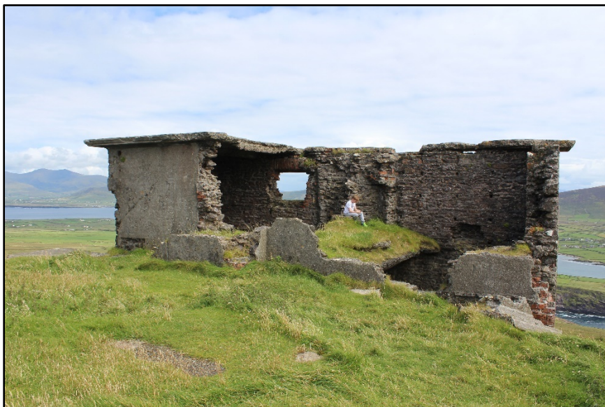
Figure F.31. View of the rear, north-west, wall of the two storey building at Sybil Head Signal Station, County Kerry, looking south-east. (Photograph courtesy of Dr James Bonsall).
