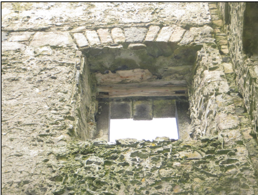
Figure A.56. First floor window on the north-west wall showing surviving parts of the timber framing.
