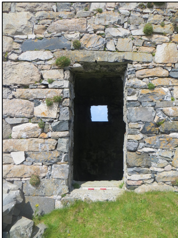
Figure A.62. Detail of the ground floor window on the south-east wall which had been converted into a neat ground level door.
