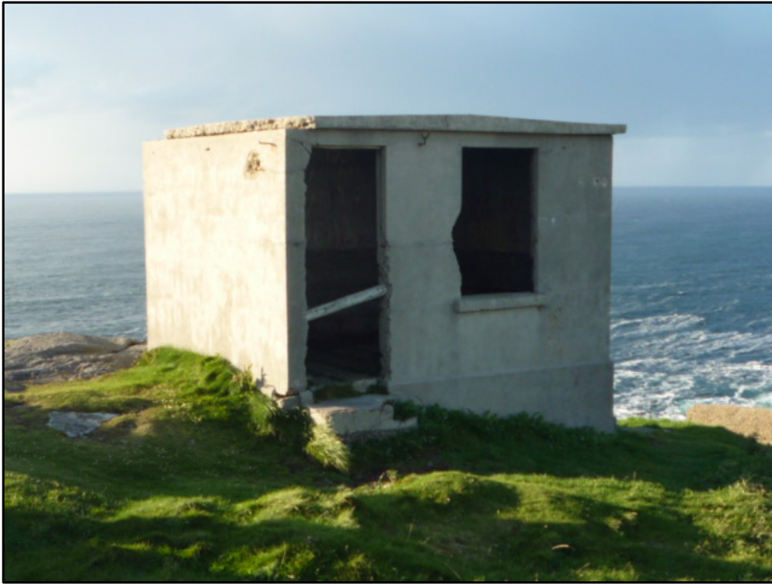
Figure D.123. The ancillary building located within the poured concrete enclosure, to the north of the signal tower at Malin Head Signal Station.
