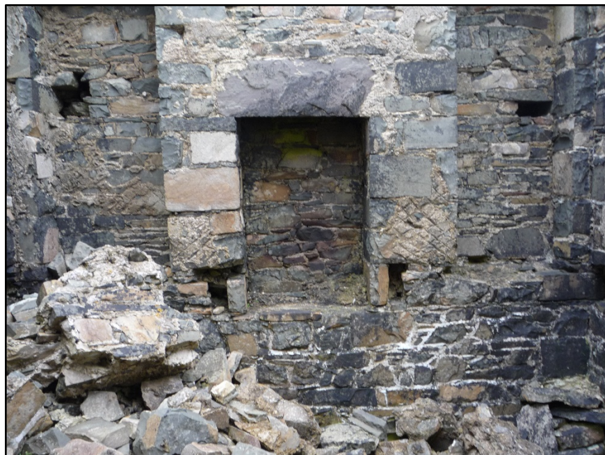
Figure B.22. The lower part of the internal face of the east wall, showing the fireplace and the bottom of the flanking alcoves.
