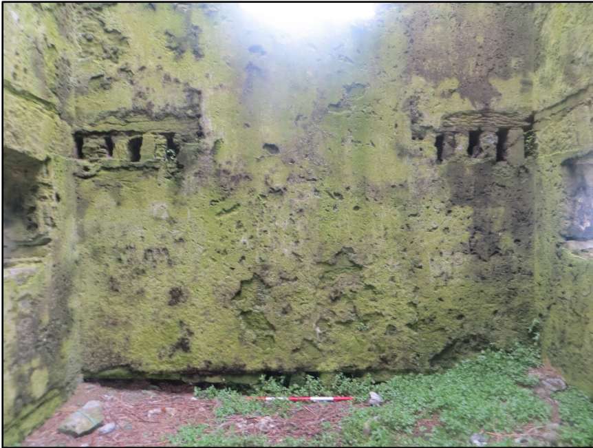
Figure A.11. The ground floor level of the internal face of the south-west wall, showing the two sets of joist holes from the split mezzanine level and the base of the first floor doorway.
