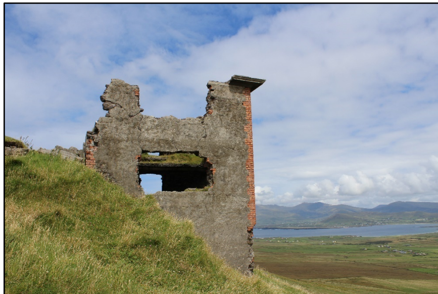
Figure F.29. View of the south-west side wall of the two storey building at Sybil Head Signal Station, County Kerry, looking north-east. (Photograph courtesy of Dr James Bonsall).
