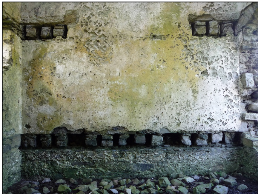
Figure C.42. The lower portion of the internal wall face of the north wall of the signal tower at Carrowmably Signal Station. The semi-basement level, the ground floor slot with joist holes, and the joist holes of the split mezzanine level can be seen.
