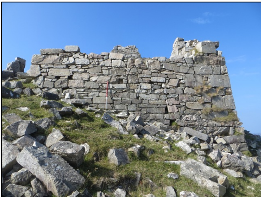
Figure A.90. The surviving portion of the external face of the east wall of the collapsed signal tower at Cleggan Hill Signal Station.
