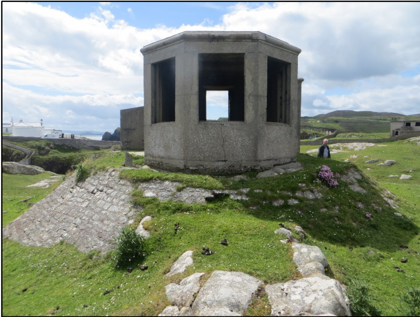
Figure D.107. The bay window on the north end of the early 20th Century watch house associated with Fanad Head Coast Guard Station.
