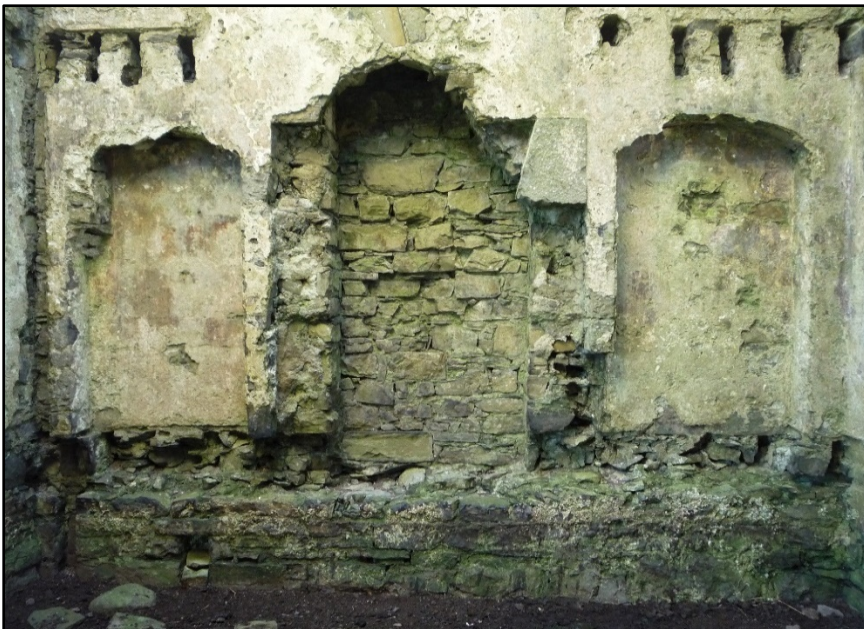
Figure C.40. The lower portion of the internal wall face of the south wall of the signal tower at Carrowmably Signal Station. The upper part of the semi-basement level, the chute into the semi-basement level, the ground floor slot, the ground floor central fireplace flanked by alcoves, and the joist holes for the split mezzanine level can be seen.
