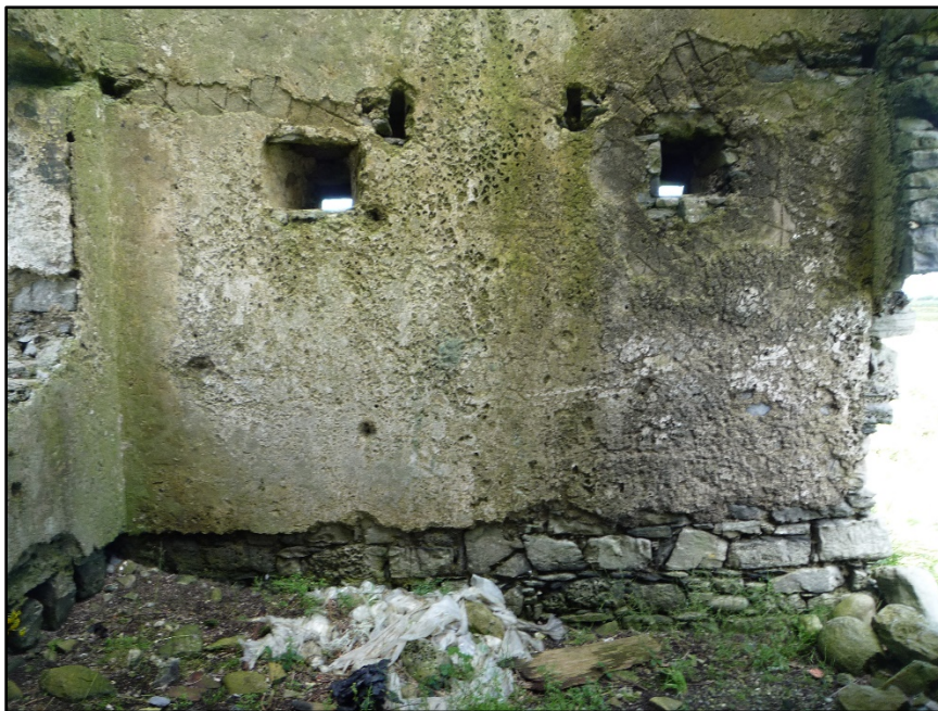
Figure C.21. The lower part of the internal face of the north wall of the signal tower at Rathlee Signal Tower. The gap in the render for the ground floor, the two square holes passing through the wall and the sloping gaps in the render connecting to the narrowly spaced joist holes that may have held the split mezzanine levels can be seen.
