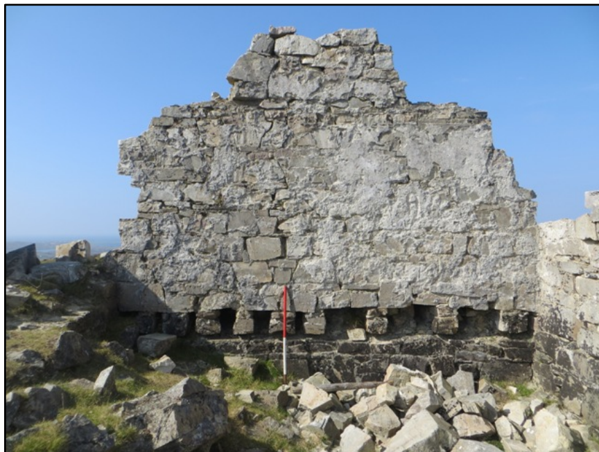
Figure A.92. The internal face of the west wall of the collapsed signal tower at Cleggan Hill Signal Station.
