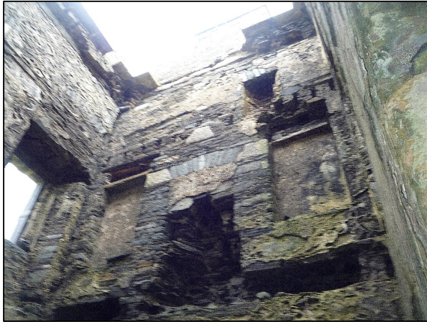
Figure D.27. The upper portion of the north-east internal wall face of the signal tower at Carrigan Head Signal Station. The position of the first floor, the first floor fireplace with flanking alcoves, the joist holes of the attic level and the unusual alcove in the attic level are visible. Note the flat stones projecting inwards from the base of the parapet level.
