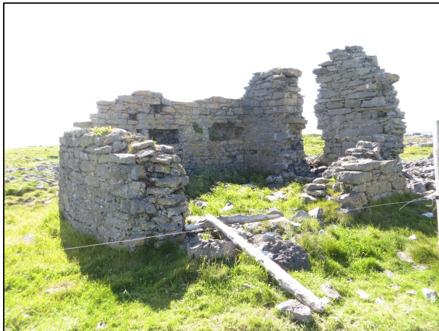
Figure C.6. View of the east corner of the collapsed or unfinished signal tower at Lenadoon Point Signal Station.
