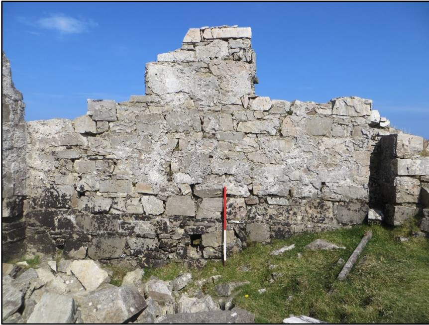
Figure A.93. The internal face of the north wall of the collapsed signal tower at Cleggan Hill Signal Station.
