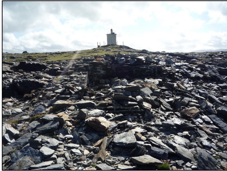
Figure D.50. The collapsed signal tower at Dawros Head Signal Tower, looking south-east, with the automated weather station in the background.
