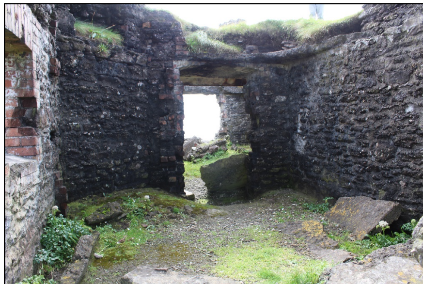
Figure F.26. Ground floor level cross wall, looking south-west. (Photograph courtesy of Dr James Bonsall).
