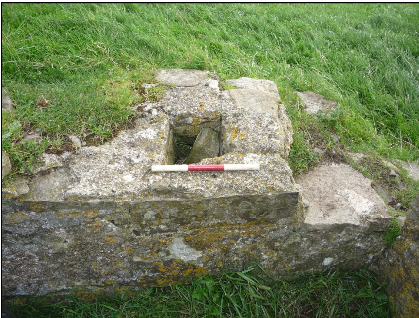
Figure C.67. Detail of the square section channel running vertically through the west corner of the collapsed signal tower at Knocklane Hill Signal Station.
