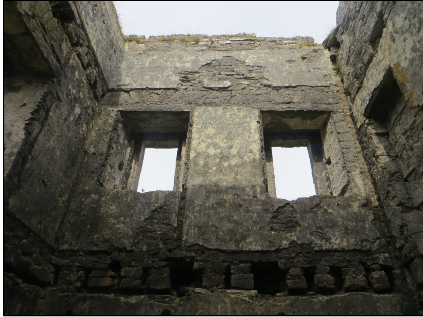
Figure A.32. The upper part of the internal wall face of the north-west wall, showing the joist holes of the first floor, the first floor windows, the impression of the attic level and the reduced parapet wall.
