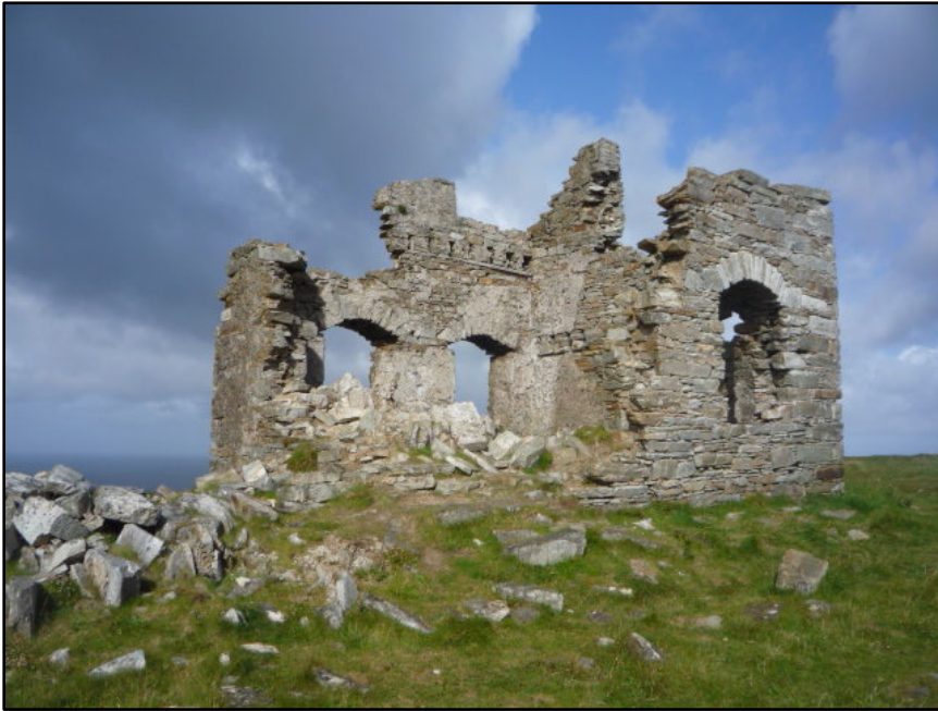
Figure D.91. View of the largely demolished south-east corner of the signal tower at Horn Head Signal Station, looking north-west.
