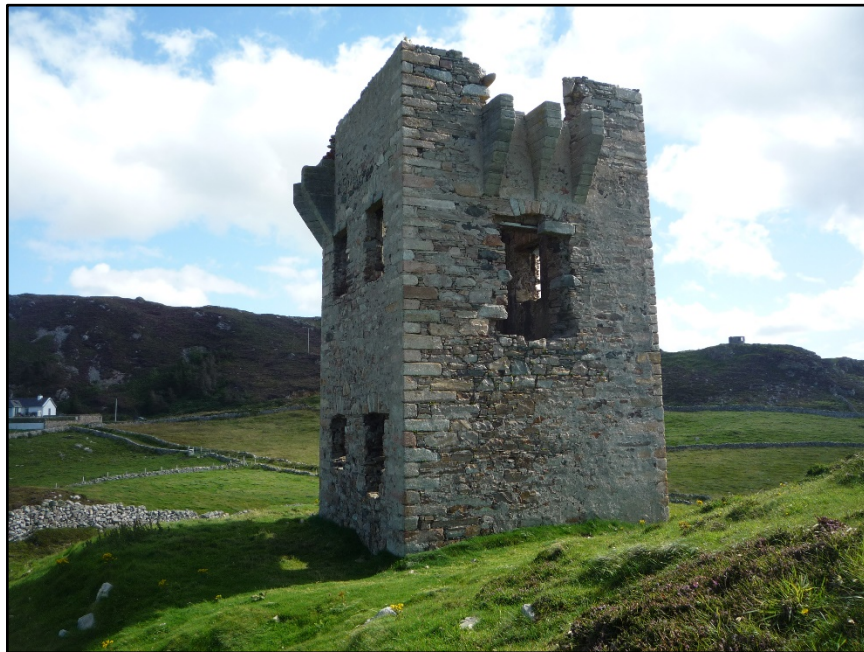
Figure D.58. The north corner of the signal tower at Crohy Head Signal Station. L.O.P. 74 can be seen on the hill top in the background, to the right of the signal tower.
