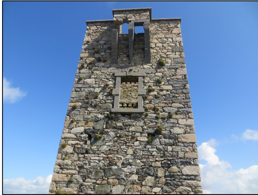
Figure A.53. The upper portion of the south-west wall of the signal tower at Golam Head Signal Station, showing the first floor door with its intact stone surround, the machicolation and the coping stones on top of the wall.
