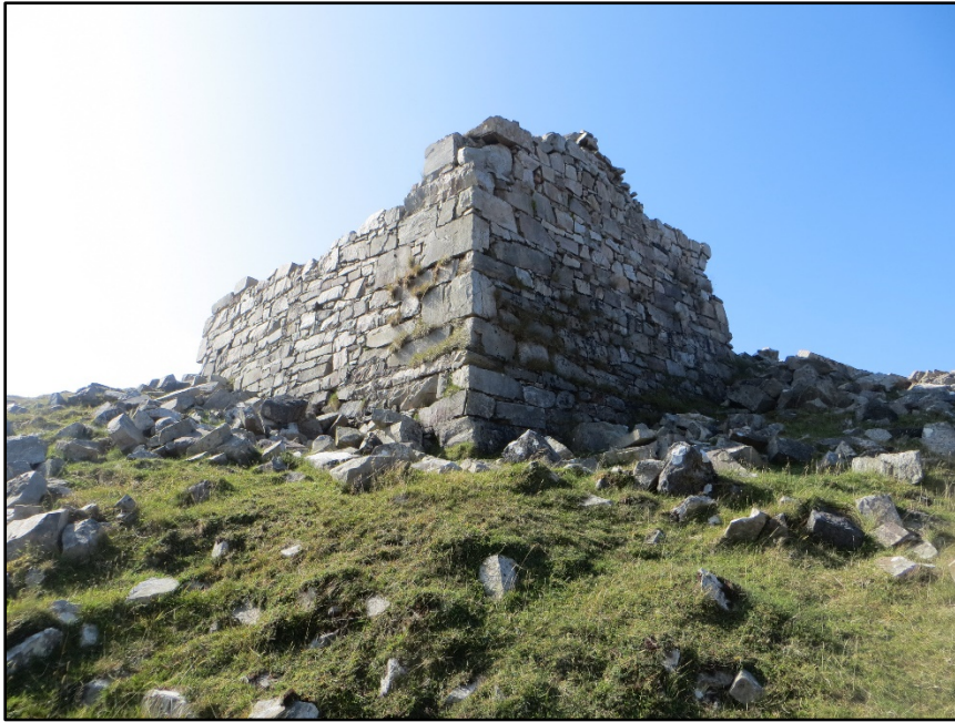
Figure A.89. View of the north-east corner of the of the collapsed signal tower at Cleggan Hill Signal Station.
