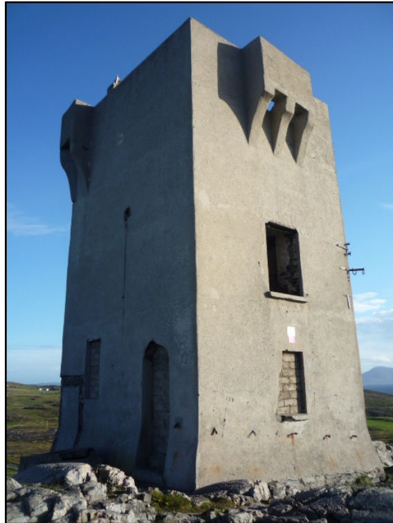
Figure D.119. The north corner of the modified signal tower at Malin Head Signal Station.
