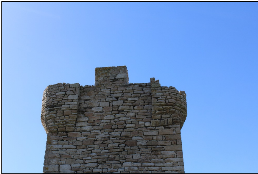
Figure B.55. The upper part of the external face of the east wall of the signal tower at Glash Signal Station, showing the curved bartizans and the well-preserved chimney.
