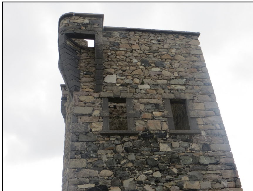
Figure A.54. The upper portion of the north-west wall of the signal tower at Golam Head Signal Station, showing the first floor windows with their intact stone surrounds, the northern bartizan and the coping stones on top of the wall.
