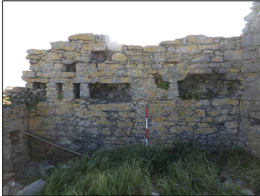
Figure C.9. View of the internal face of the south-west wall of the collapsed or unfinished signal tower at Lenadoon Point Signal Station.
