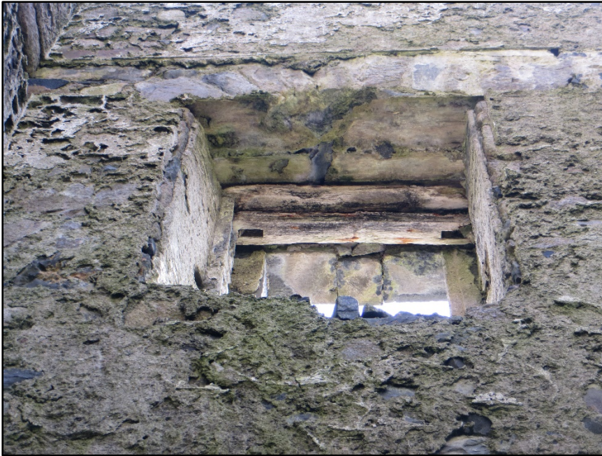
Figure A.55. First floor window on the south-east wall, showing surviving parts of the timber framing and the square holes cut into the splayed sides.
