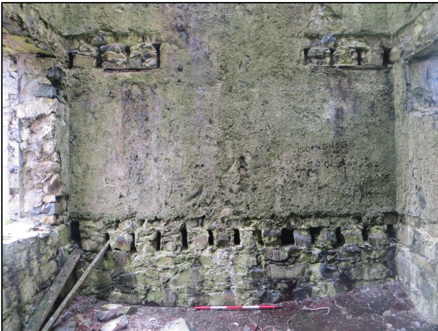
Figure A.60. The lower portion of the internal face of the south-west wall, showing the joist holes of the ground floor level and the joist holes of the split mezzanine level.
