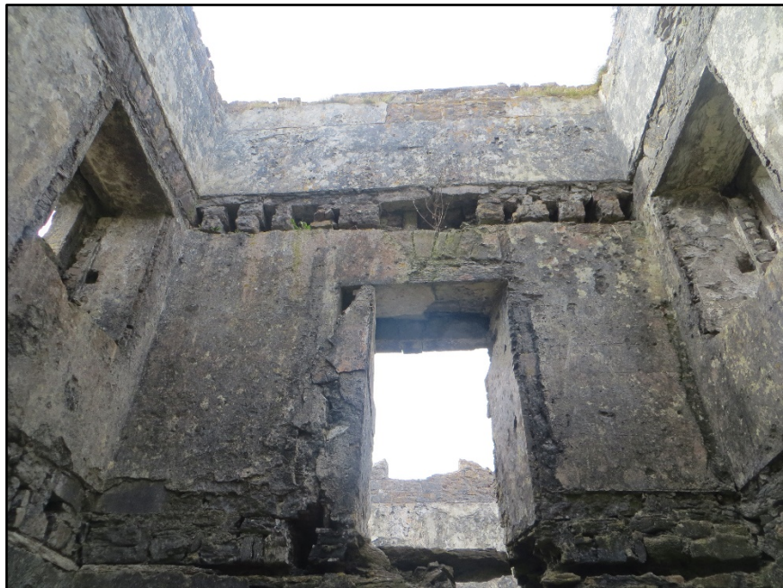
Figure A.33. The upper part of the internal wall face of the south-west wall, showing the first floor door, the joist holes of the attic level and the reduced parapet wall.
