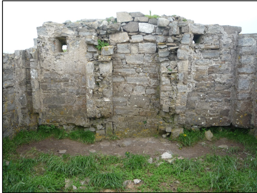
Figure C.64. Internal face of the south-east wall of the collapsed signal tower at Knocklane Hill Signal Station. The central fireplace, the flanking alcoves, the chutes passing through the wall at the top of the alcoves, and the vertical drainage channel at the north corner of the wall can be seen.
