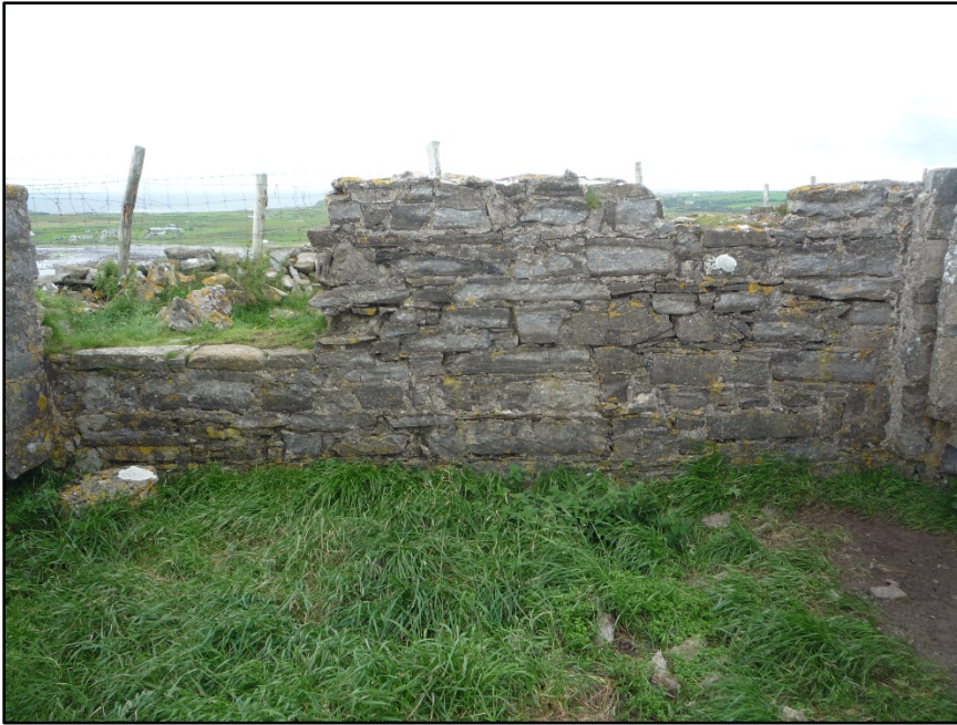
Figure C.66. Internal face of the north-east wall of the collapsed signal tower at Knocklane Hill Signal Station.
