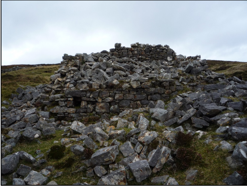
Figure B.82. The external face of the south wall of the collapsed signal tower at Glinsk Signal Station. The chute passing through the wall is visible towards the left.
