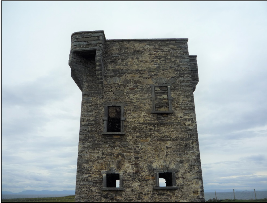
Figure D.25. The upper portion of the north-west external wall of the signal tower at Carrigan Head Signal Station, showing the repositioned north window, the infilled south window, the north bartizan and the ground floor windows.
