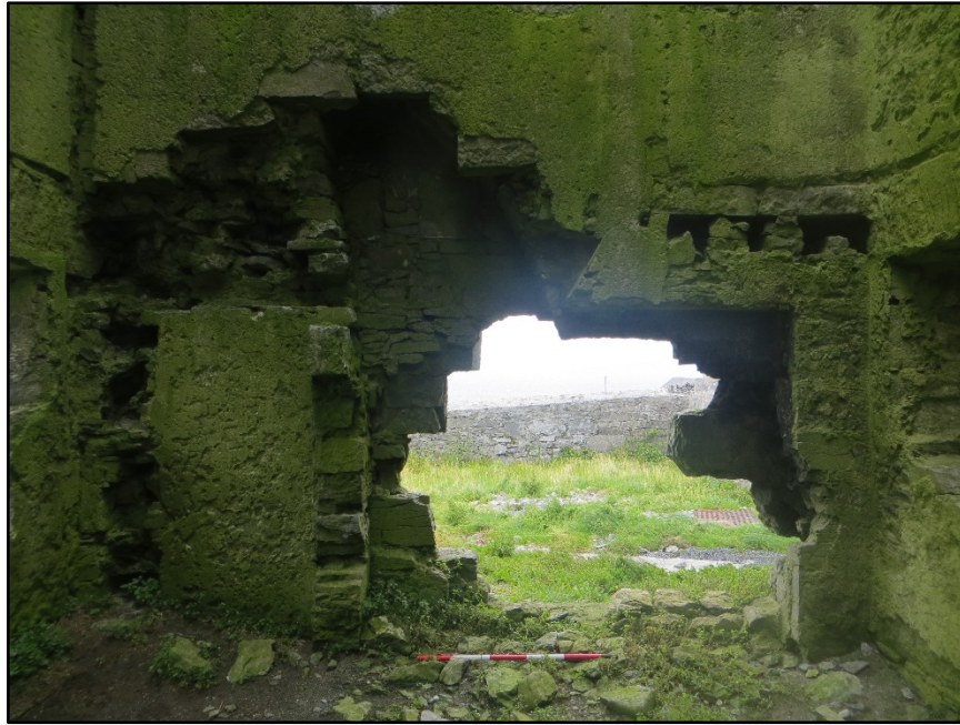
Figure A.9. The damaged area of the ground floor level of the internal face of the north-east wall. The damaged alcoves can be seen at either side and the curving flue that would have connected to the largely removed fireplace can be seen. The row of joist holes from the south-east mezzanine level can be seen at the right of the wall.
