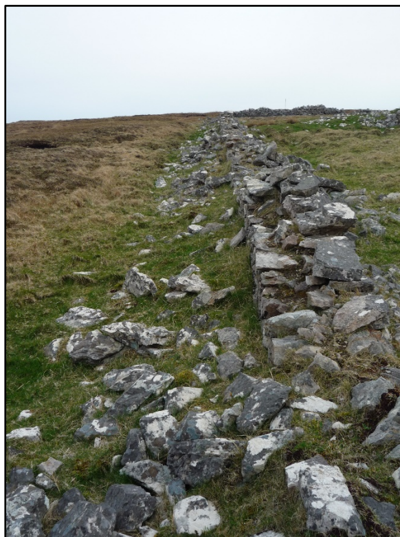
Figure B.71. Detail of the perimeter of the north-east side of the enclosure, looking south-east, showing the collapsed wall and the external ditch.
