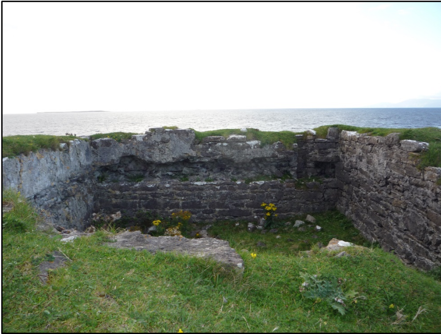
Figure C.75. The internal north-west wall face of the collapsed signal tower at Streedagh Signal Station.
