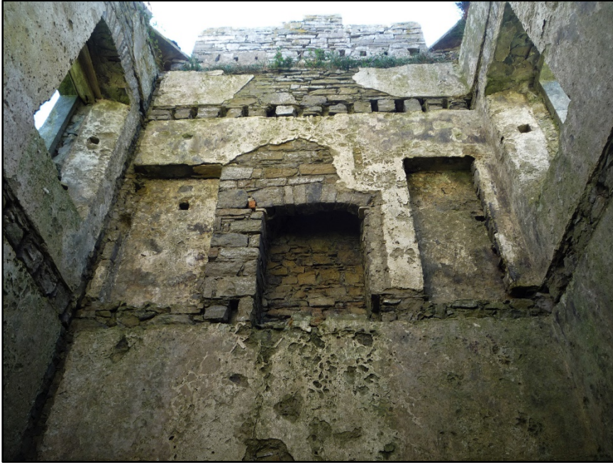
Figure C.39. The upper portion of the internal wall face of the south wall of the signal tower at Carrowmably Signal Station. The first floor fireplace and flanking alcoves, the attic level slot, the instep at the parapet level, the roof level joist holes, the entrances to the bartizans and the drainage channel running down the southern edge of the east wall can be seen.
