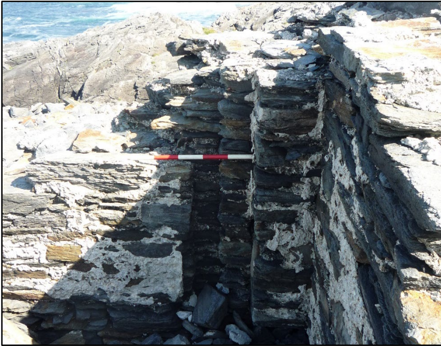
Figure D.52. Detail of the surviving portion of the vertical drainage channel at the south-east of the north-east internal wall face of the collapsed signal tower at Dawros Head Signal Station.
