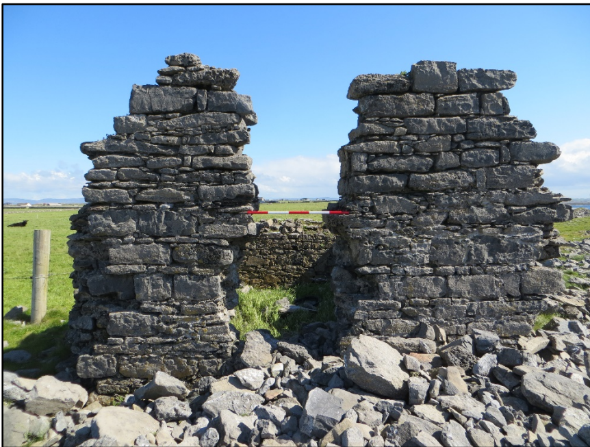
Figure C.8. View of the external face of the north-west wall of the collapsed or unfinished signal tower at Lenadoon Point Signal Station.
