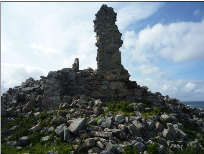
Figure D.100. The external face of the east wall of the collapsed signal tower at Melmore Head Signal Station, showing the surviving stonework that appeared to have been the pillar that separated the ground floor windows, and the external buttress at the south of the wall.
