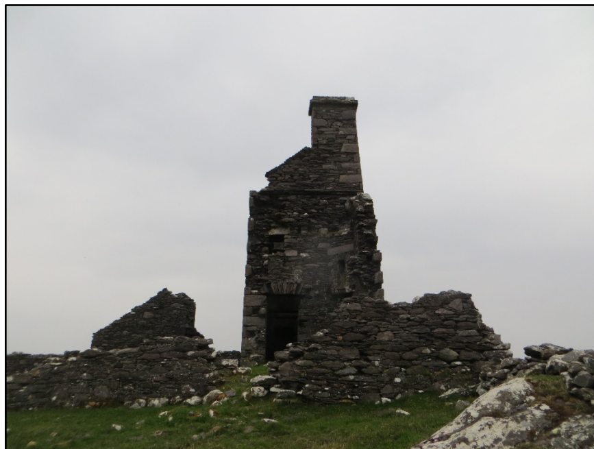
Figure G.5. The southern end wall of the two storey building at Hog's Head Enclosed Barrack, County Kerry, with the collapsed addition projecting from the wall and the free-standing external stairs to the left, looking north.
