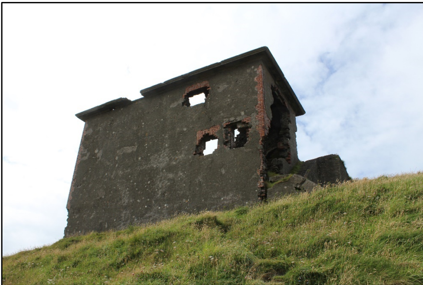
Figure F.28. View of the front, south-east, wall of the two storey building at Sybil Head Signal Station, County Kerry, looking north-west. (Photograph courtesy of Dr James Bonsall).
