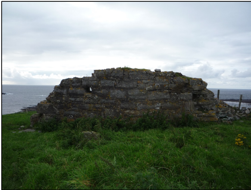
Figure C.62. External face of the south-east wall of the collapsed signal tower at Knocklane Hill Signal Station.
