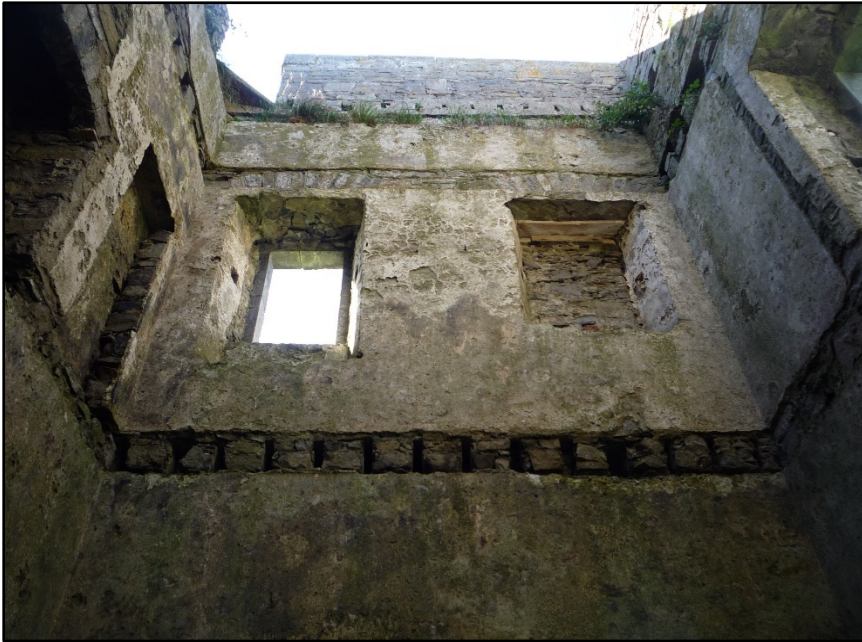
Figure C.43. The upper portion of the internal wall face of the south wall of the signal tower at Carrowmably Signal Station. The slot with joist holes for the first floor, the open south window with square bar hole, the north blocked window with square bar hole and timber frame parts, the attic level slot, the parapet wall, the parapet wall joist holes and the entrance to the south-west bartizan are visible.
