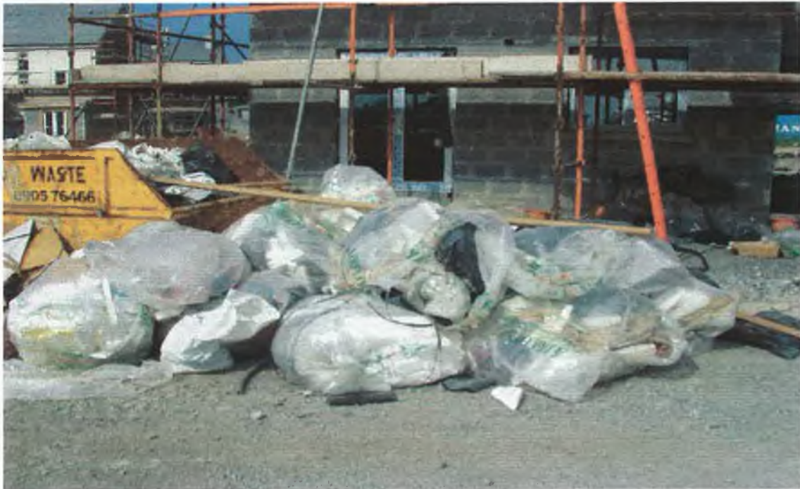
Photo 6.5 Build Up of Site Wastes
