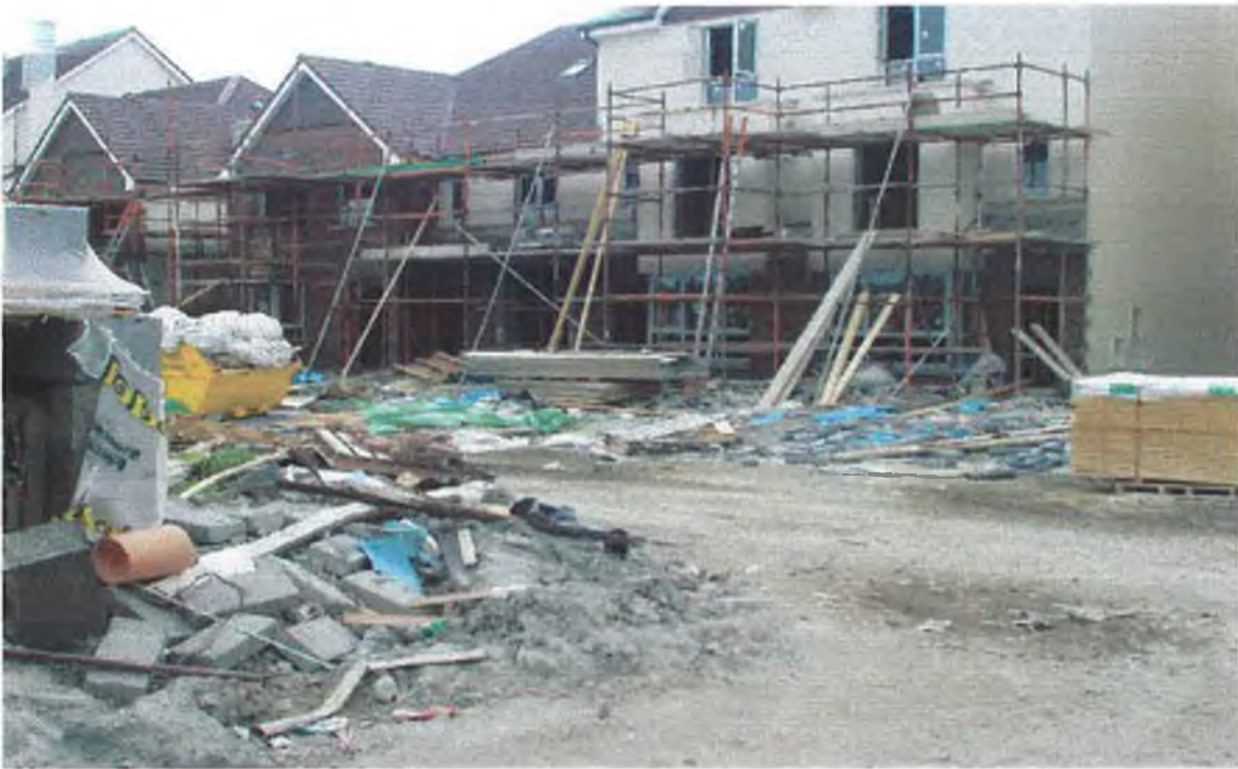
Photo 3.2 The build-up of site wastes around scaffolding can be excessive.
