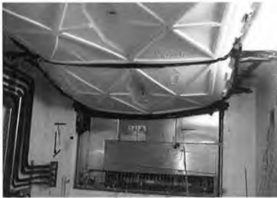
Figure 2-25: Duct fitted to TK refrigeration unit
