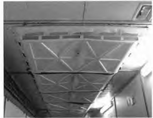
Figure 2-26: The end of the duct
