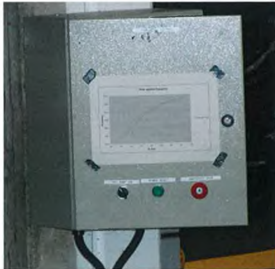
Figure 3-21: Speed drive control box used to control the pump speed
