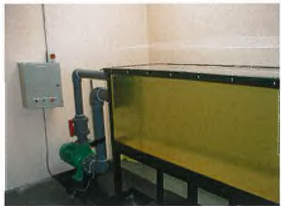
Figure D-4: The attachment of the pump to the tank and the speed drive
