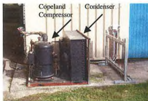
Figure 3. 6 Externally Outside located condensing unit for calibrated box cooling system.
