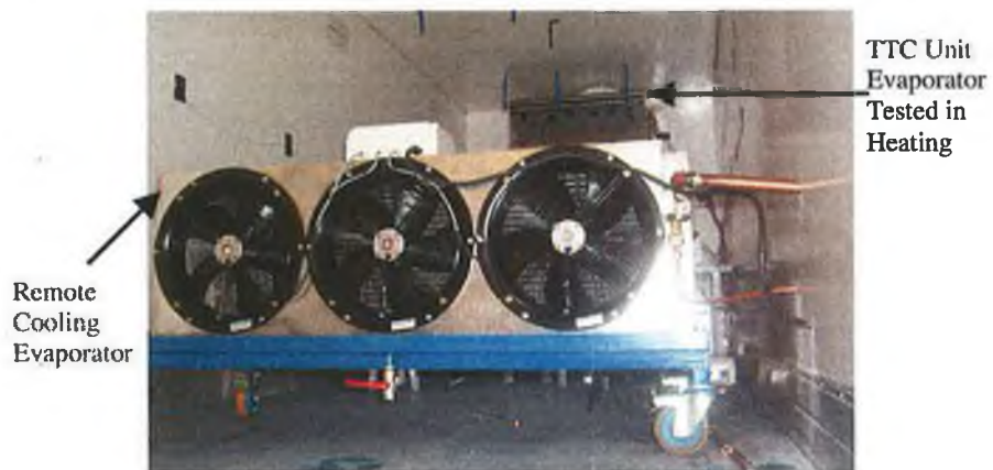
Figure 3.7 Remote Evaporator located inside the calibrated box.
