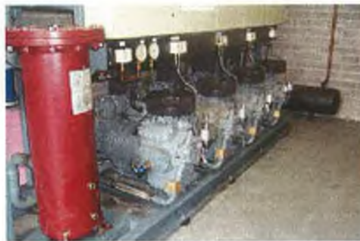
Figure F.1 Ambient Room main compressors (Item 4, Figure 3.3).
