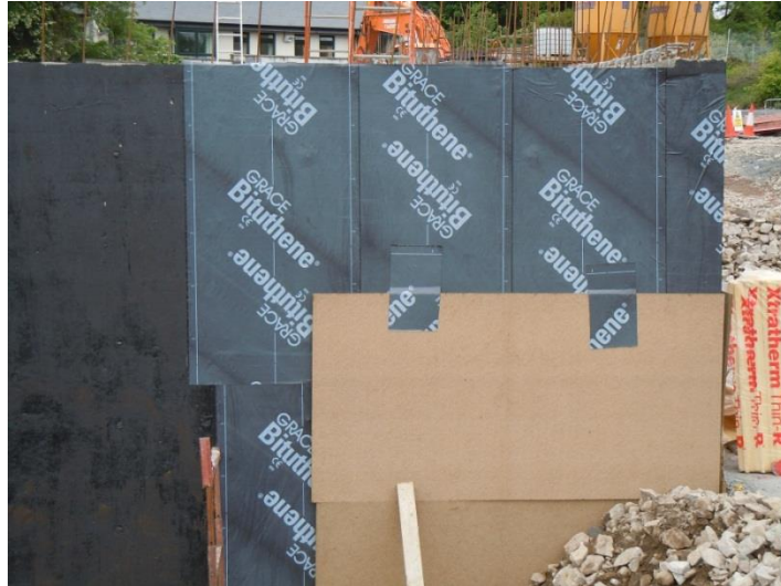
Picture 6.68 Inappropriate use of materials
