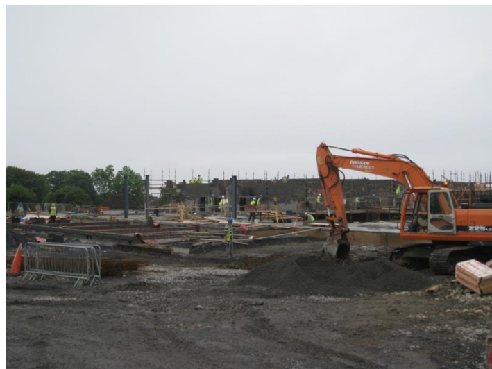
Picture 6.39 Wastage of concrete 1
