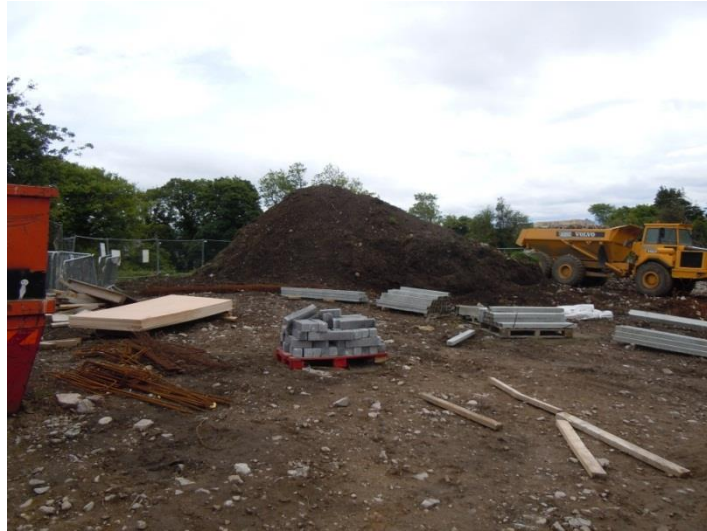
Picture 6.18 Incorrect storage of topsoil
