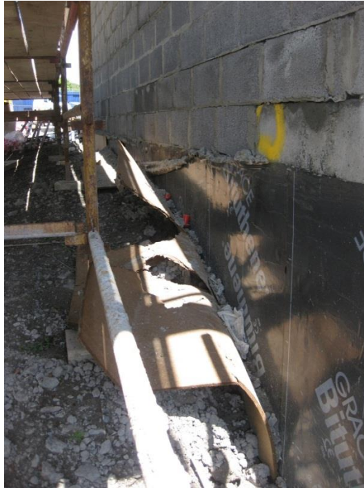
Picture 6.73 Poor installation of materials 1
