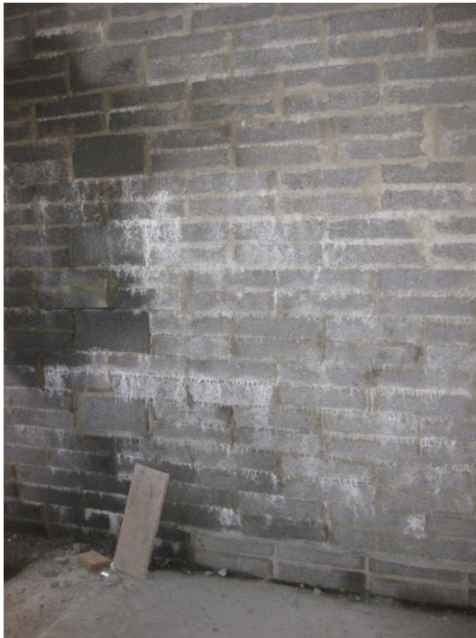
Picture 6.79 Efflorescence on block work
