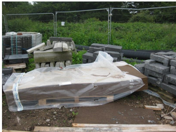
Picture 6.29 Poor storage of protection barrier
