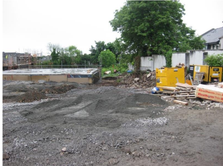
Picture 6.40 Wastage of concrete 2
