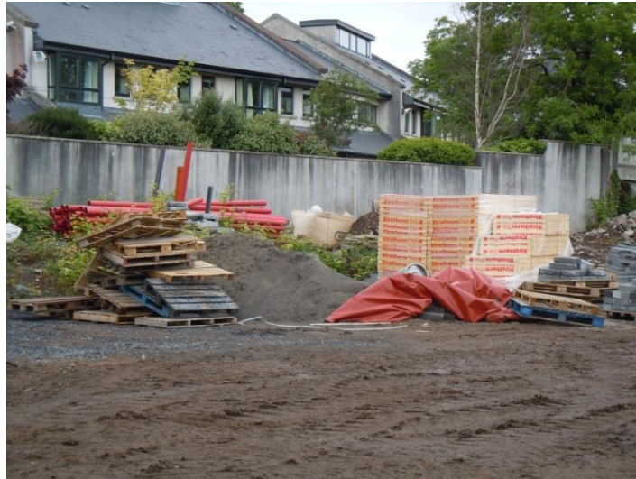
Picture 6.15 Inadequate storage of sand
