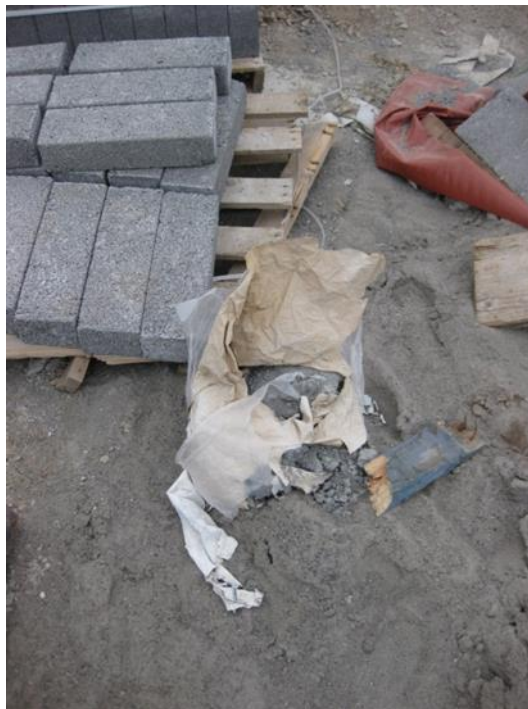
Picture 6.26 Poor storage of concrete bags
