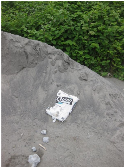
Picture 6.25 Poor storage of concrete bags
