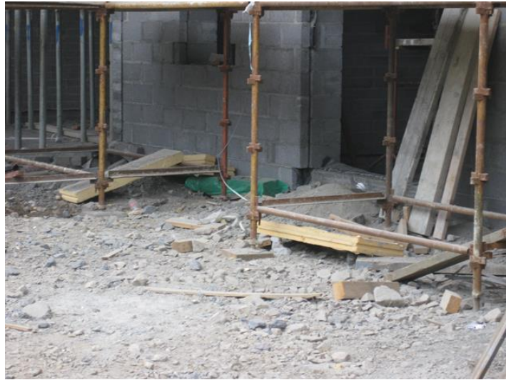
Picture 6.27 Insulation materials damaged
