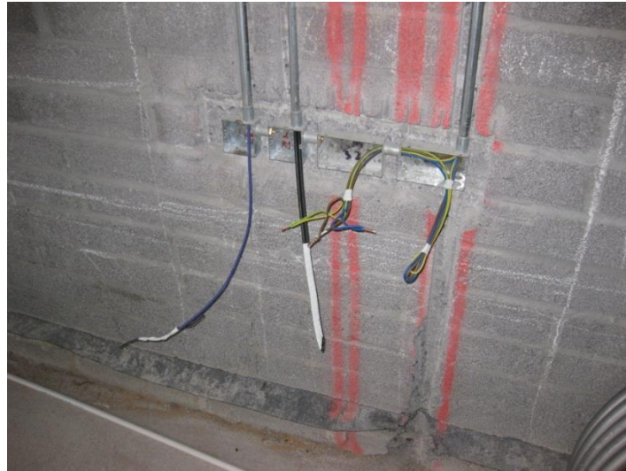
Picture 6.61 Electrical wire tails
