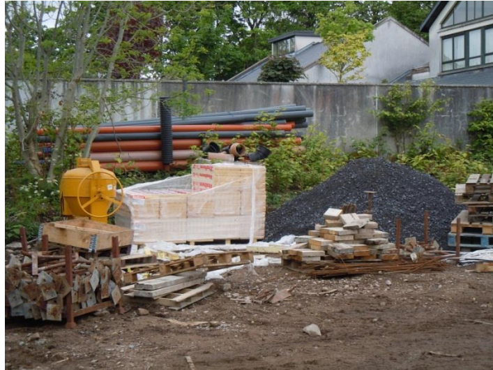
Picture 6.16 Inadequate storage of stone
