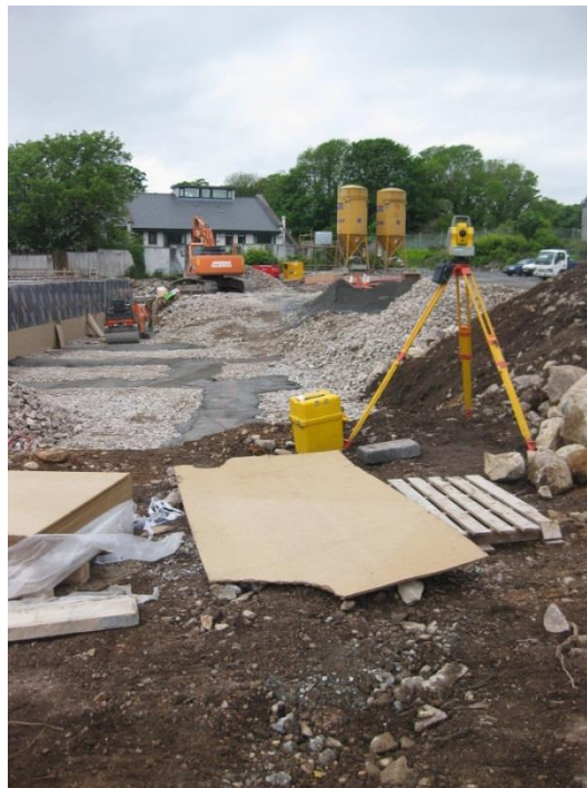
Picture 6.17 Poor storage of protection barrier
