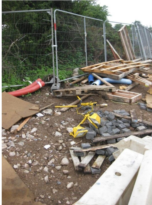
Picture 6.28 Equipment damage
