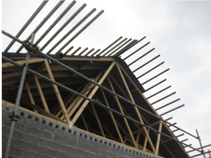
Picture 6.13 Roofing battens overruns
