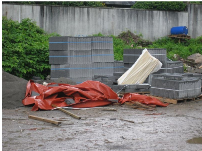
Picture 6.32 Incorrect use of materials 2
