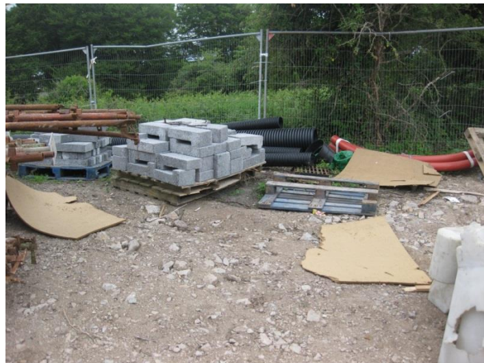
Picture 6.22 Protection barrier damage 2
