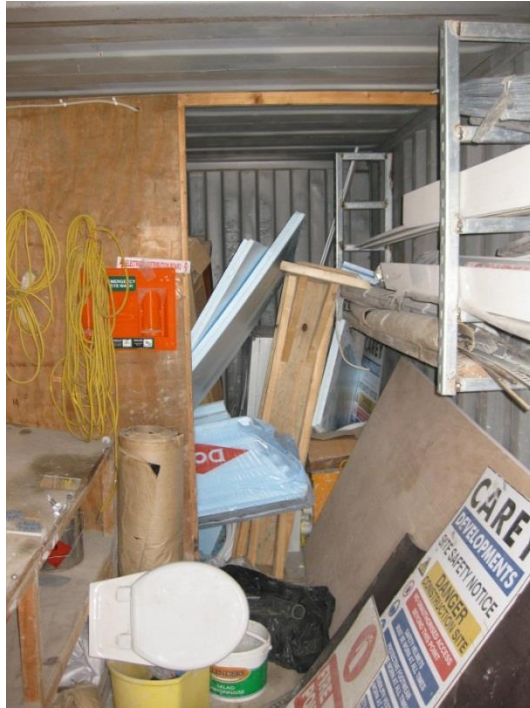
Picture 6.19 Poor storage of materials 1
