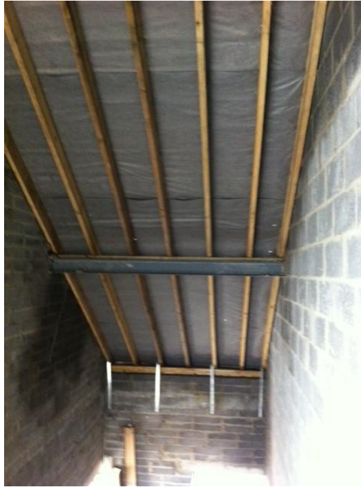
Picture 6.81 Holes in the roofing membrane
