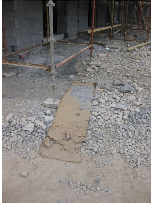
Picture 6.21 Protection barrier damage 1
