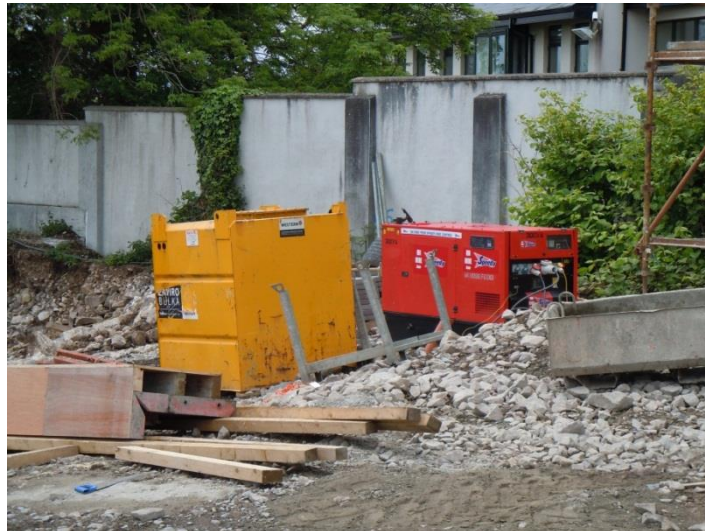
Picture 6.63 Mobile generator
