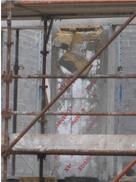
Picture 6.78 Insulation damage
