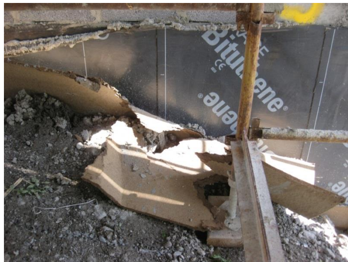
Picture 6.74 Poor installation of materials 2
