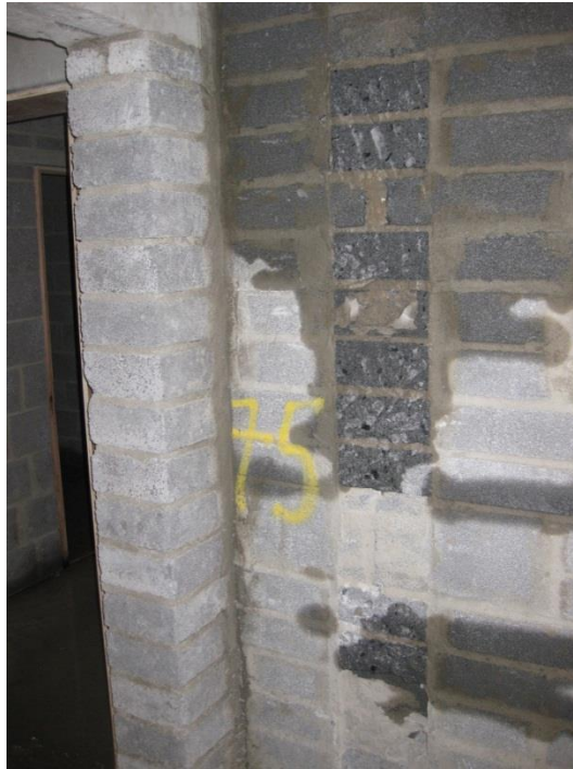
Picture 6.57 Walls built incorrectly
