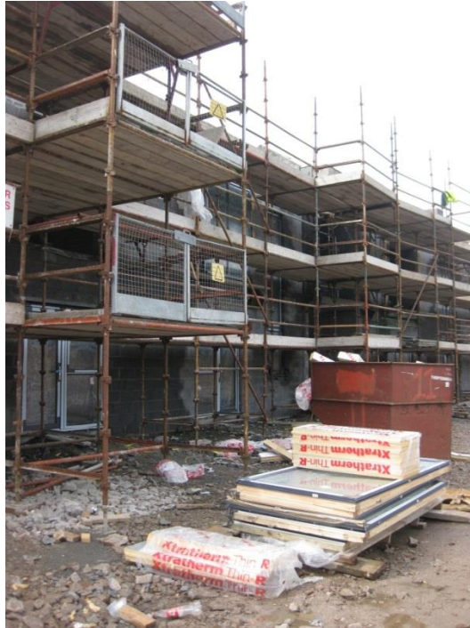
Picture 6.30 Poor storage of windows and doors
