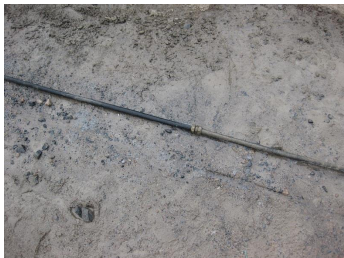
Picture 6.66 Leaking water pipe
