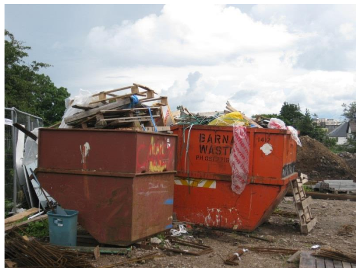
Picture 6.76 Overflowing skips
