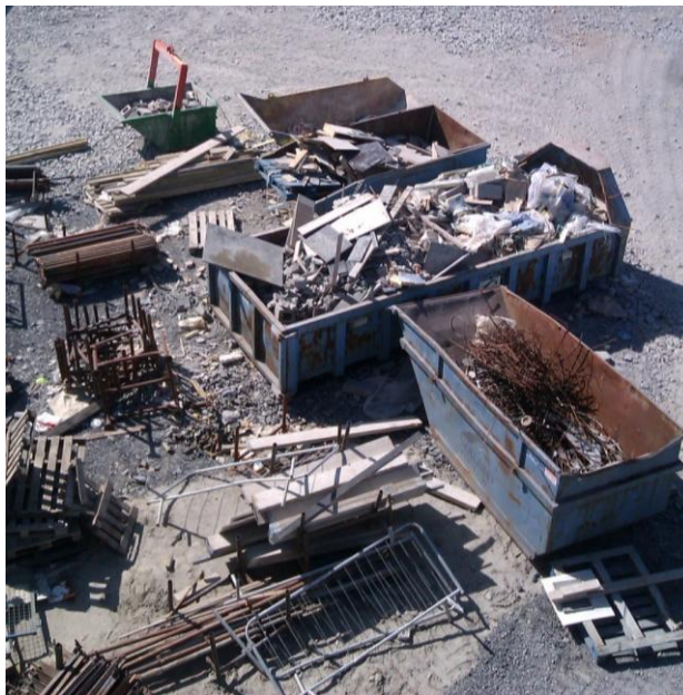
Photograph 5.4: Day 1. Large skip area - approximately 4% (Metal); 14% (Mixed); and 5% (Timber) non-compliance
