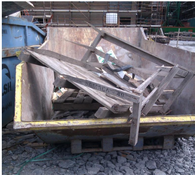
Photograph 5.20: Day 2. Timber skip B containing timber and insulation materials – approximately 10% non-compliance
