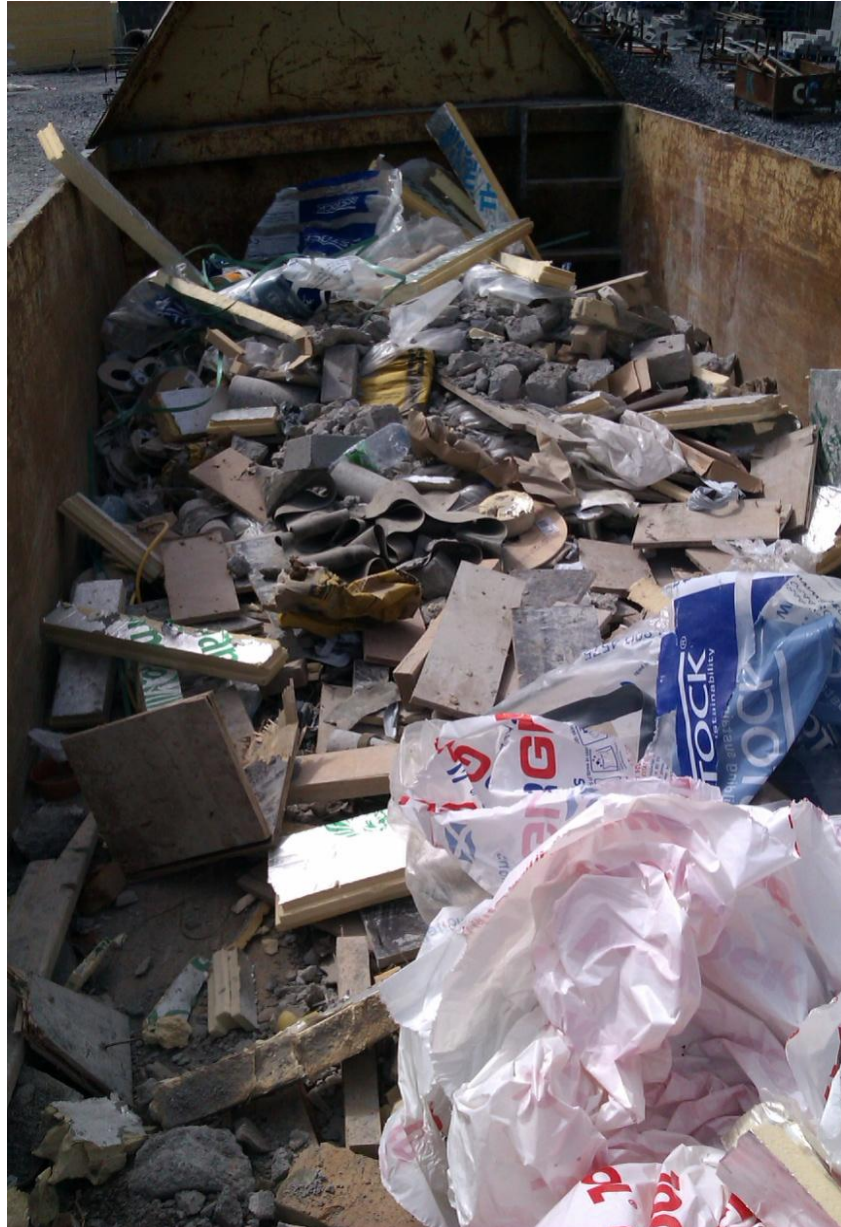
Photograph 5.36: Day 4. Mixed skip – approximately 10% non-compliance
