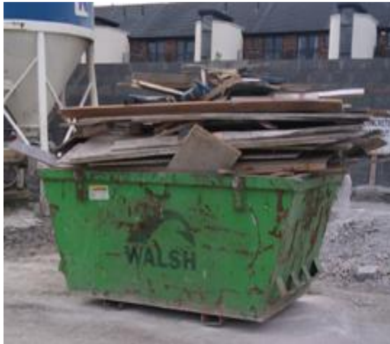
Photograph 5.19: Day 2. Full timber skip (A)– approximately 5% non-compliance
