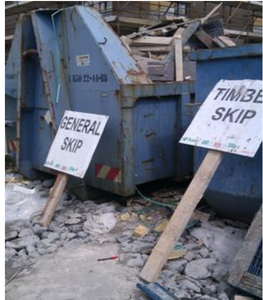
Photograph 5.16: Day 2 Poor signage – approximately 50% non-compliance
