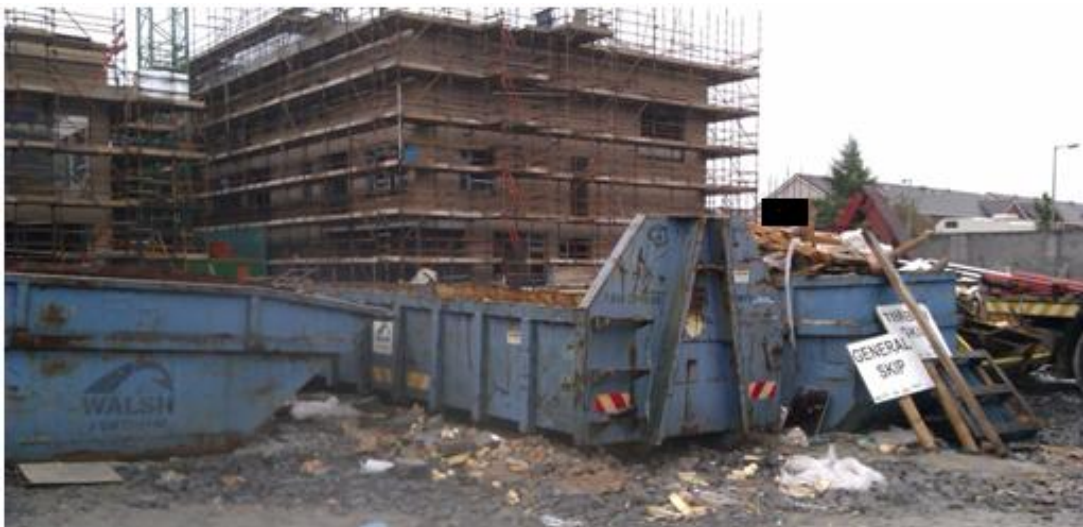
Photograph 5.28: Day 3. Empty mixed skip 2. Site worker omitted for the purposes of privacy.
