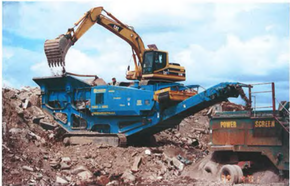
Photograph 6.1 Construction and demolition waste being transferred to the 'jaw' crusher on the DemCon 20/20 project
