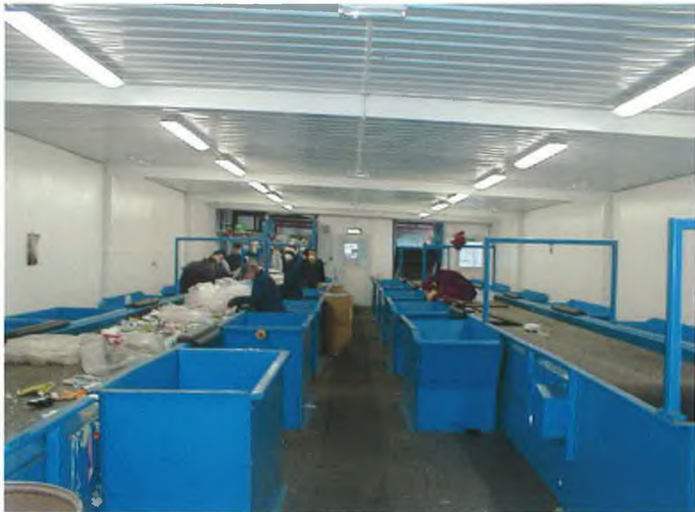
Photograph 8.7 Manual picking station in operation at the Barna Waste facility
