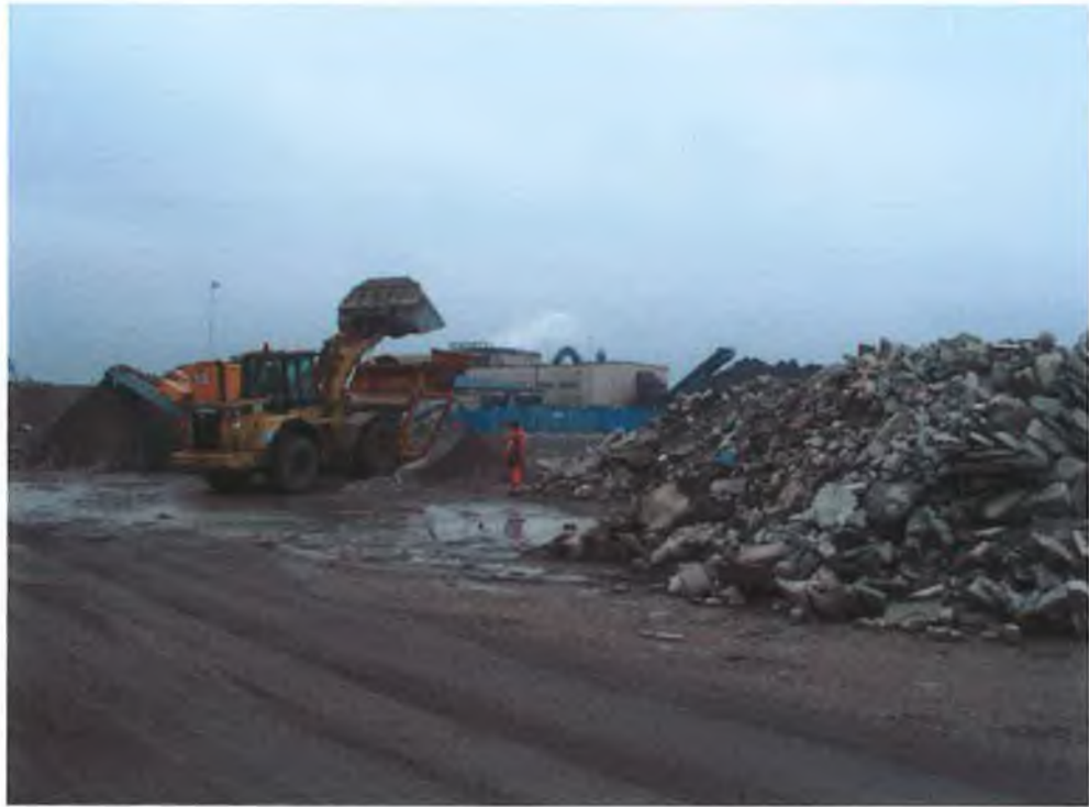
Photograph 6.16 Processing system in operation at the Spillepeng site.
