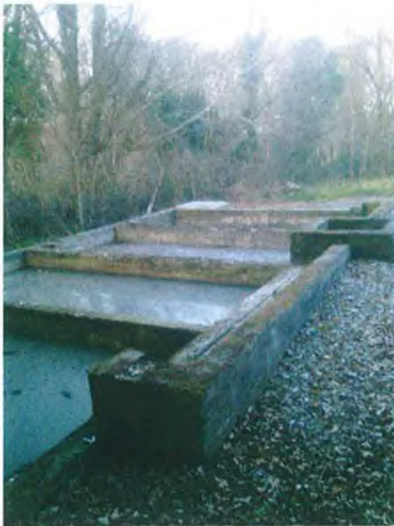
Figure 10. Treatment plant Woodford Co Galway
