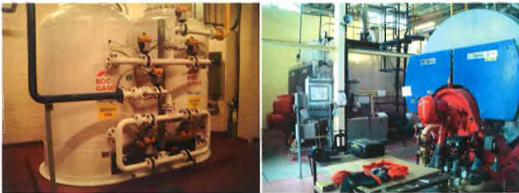
Nitrogen Pressure Swing Absorption (PSA) Plant and Gas Fuelled Boilers
