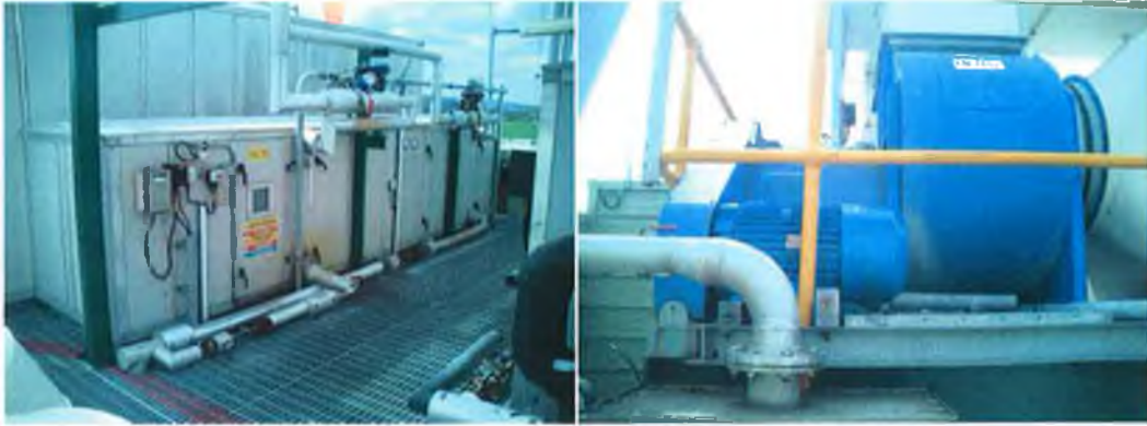
Typical Air Handling Unit and Fan (HVAC System)
