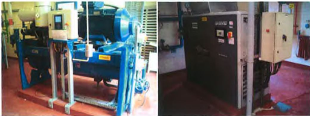
Typical Plant Air Compressor and Breathing Air Compressor
