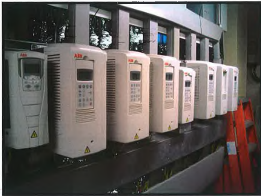
Figure 30: Eight of the Variable Speed Drive (VSD) Units Installed
