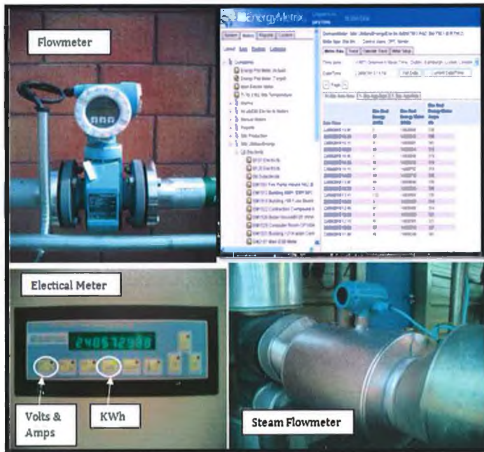
Figure 27: Energy Monitoring System & Energy Metering Devices
