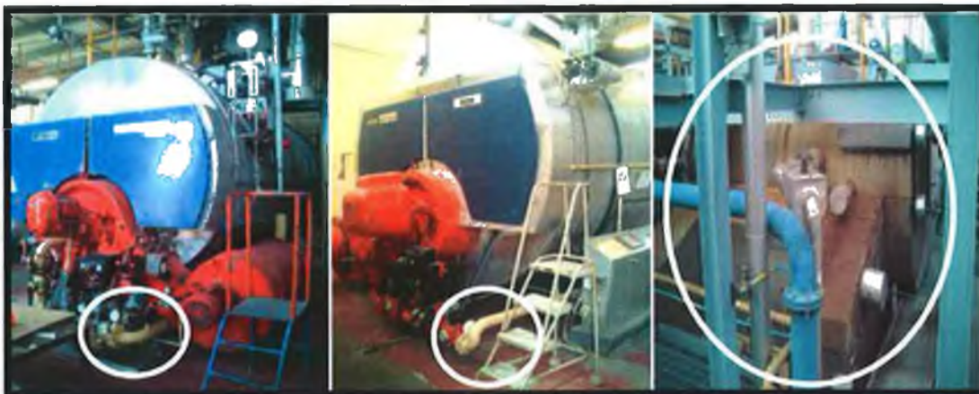
Figure 25: Boiler 2002, Boiler 2003, and Waste Heat Boiler 1931[43]
