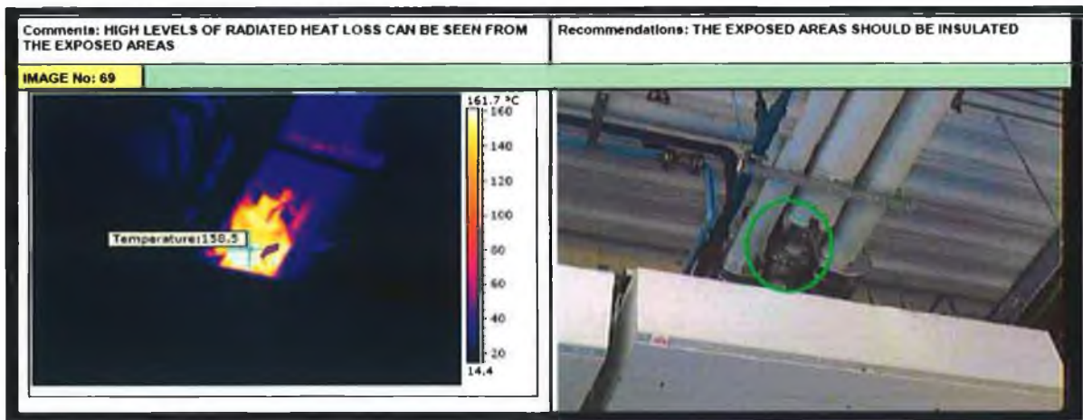
Figure 34: Exposed High Level Valve Connection
