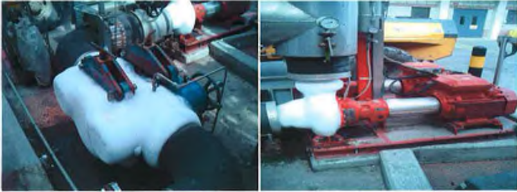
Un-insulated Refrigeration Distribution Line Filter and Pump
