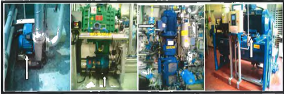
Figure 23: Examples of Motors on Site, Fan, Vacuum, Agitator and Compressor Motors [43]
