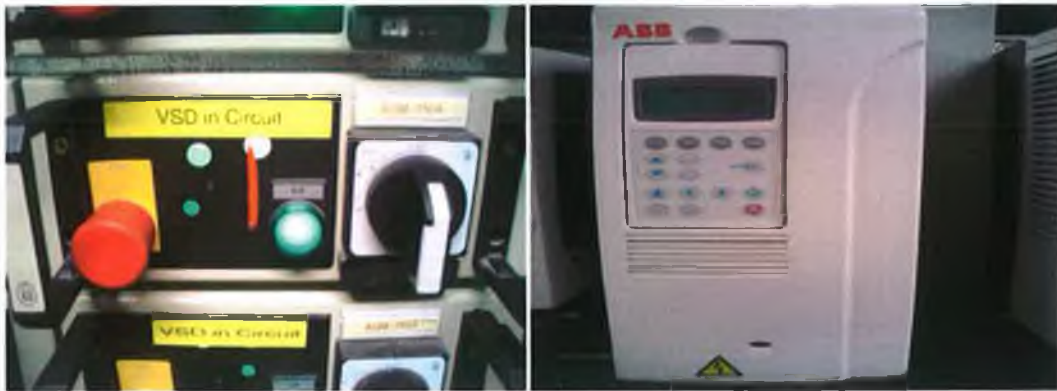
VSD MCC room plate and VSD Unit for an Agitator Motor
