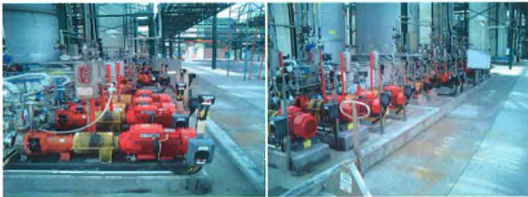
Tank Farm Pumps and Motors
