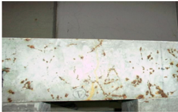
Figure 2.2 – SFRC with fibres corroded.
