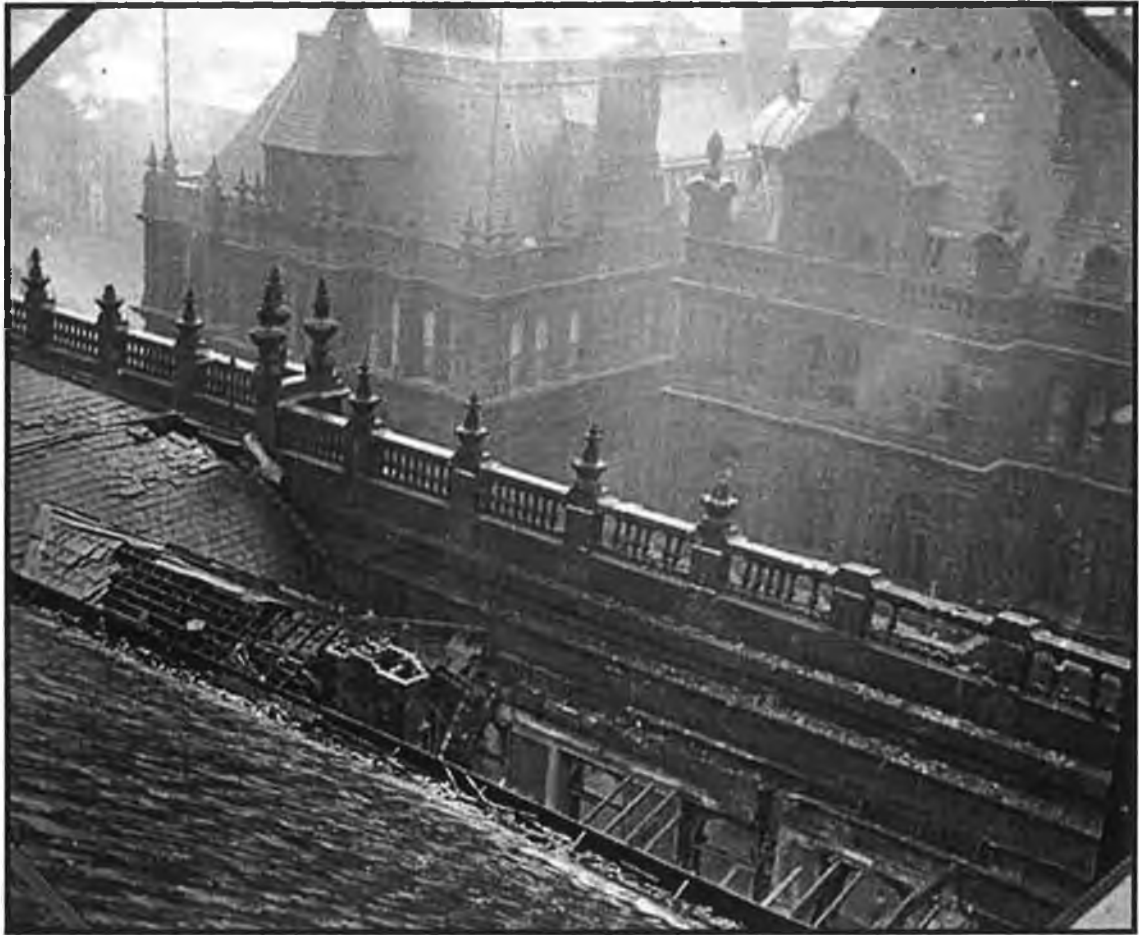
Plate 25: Roof Bomb Damage, Town Hall, The Headrow, 1941.
