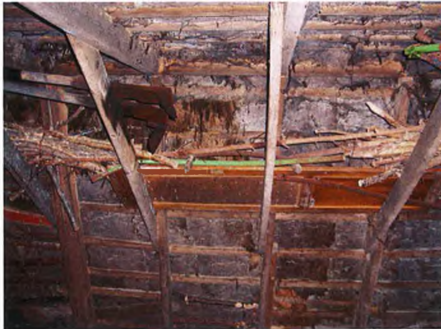
Plate 108 – The tie-beam couple truss roof structure of Ballycroy's traditional stone cottage (Figure 37).
