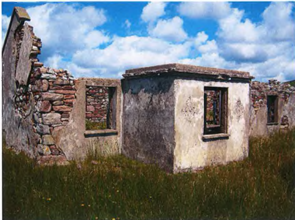
Plate 51 – Site 4, Sheeanmore, the Congested Districts Board house. Note the dry stone walling underneath the plaster which erosion is exposing.
