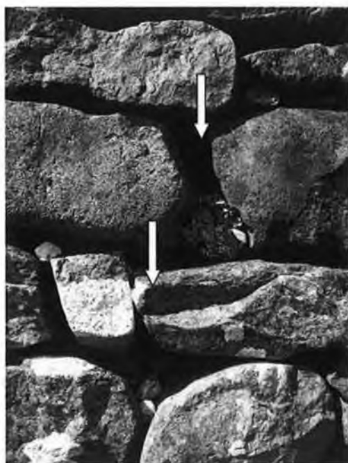
Plate 116 – Shell mortar in the stone-walls of the stone cottages in Figure 31 of this study.
