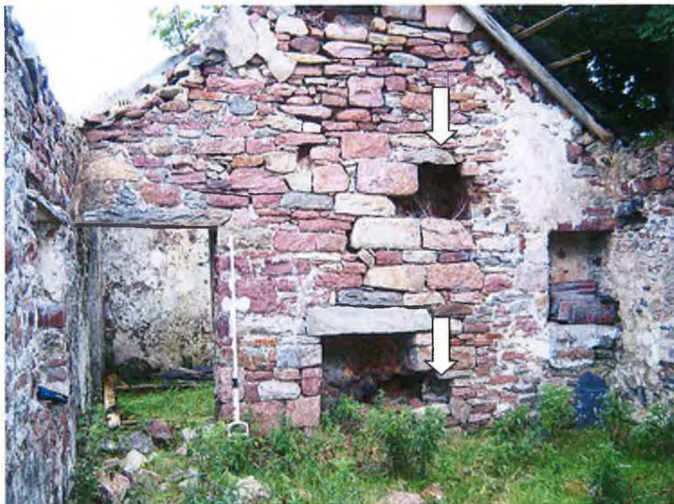
Plate 55 – The interior of the house (Figure 36 in section 4.4.1.2), note the central hearth and keeping holes in wall.
