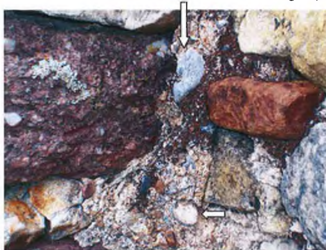
Plate 86 - Cockle and mussel shells in the sand mortar of the stone cottage (Figure 30).
