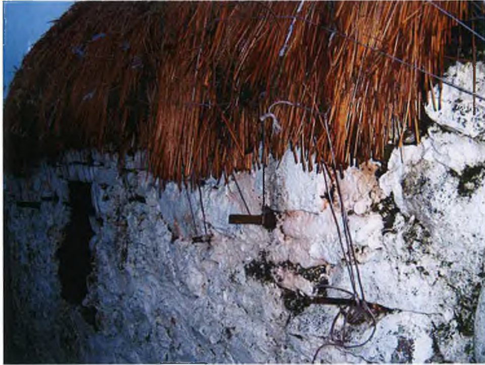
Plate 110 - Scraw wooden pegs used in the tie-beam thatching. The scraws are inserted into the stone wall.
