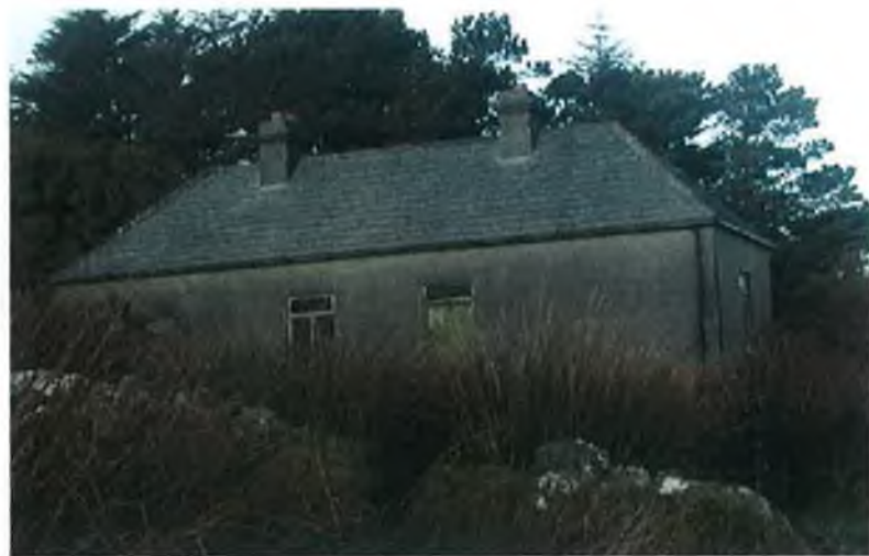
Plate 48 Derelict House Slievemore
